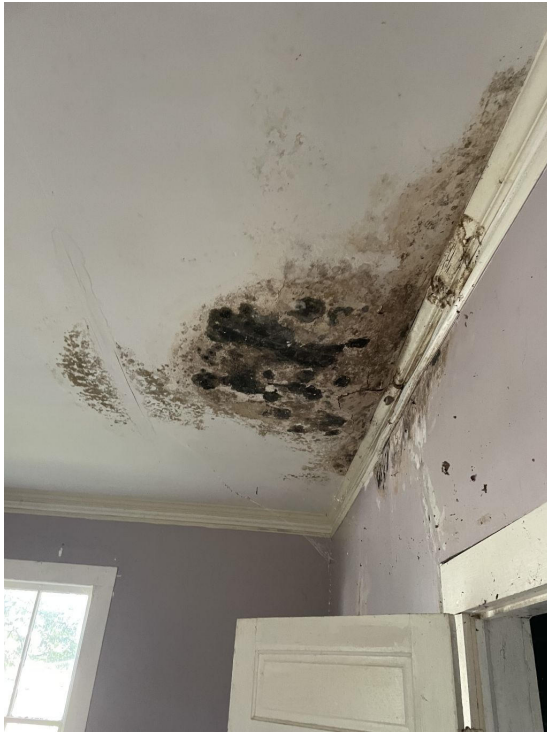
Right front room at entry door. Roof leak.
