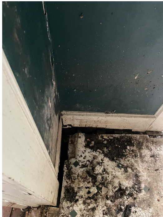
Foyer- Front Center Room at front door.. Rotted floor from water damage
