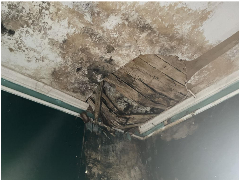
Foyer- Front Center Room at front door.. Rotted ceiling above rotted floor from water damage
