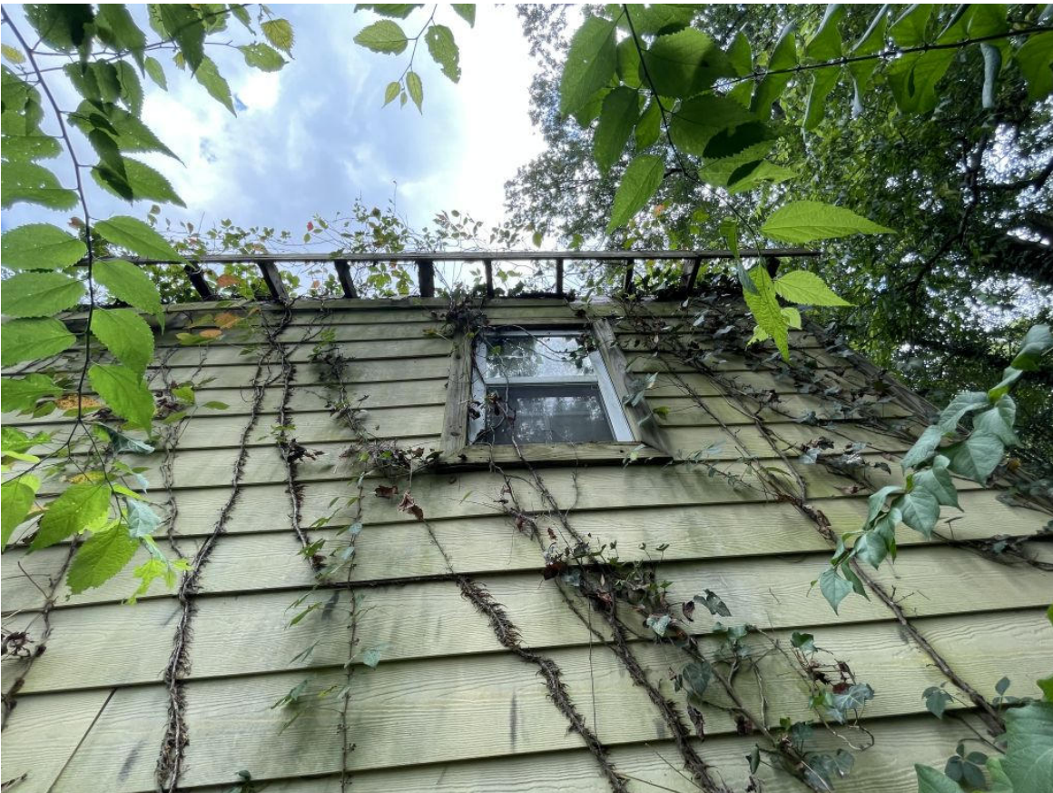
View to rear of home from SW corner. Roof missing on addition.
