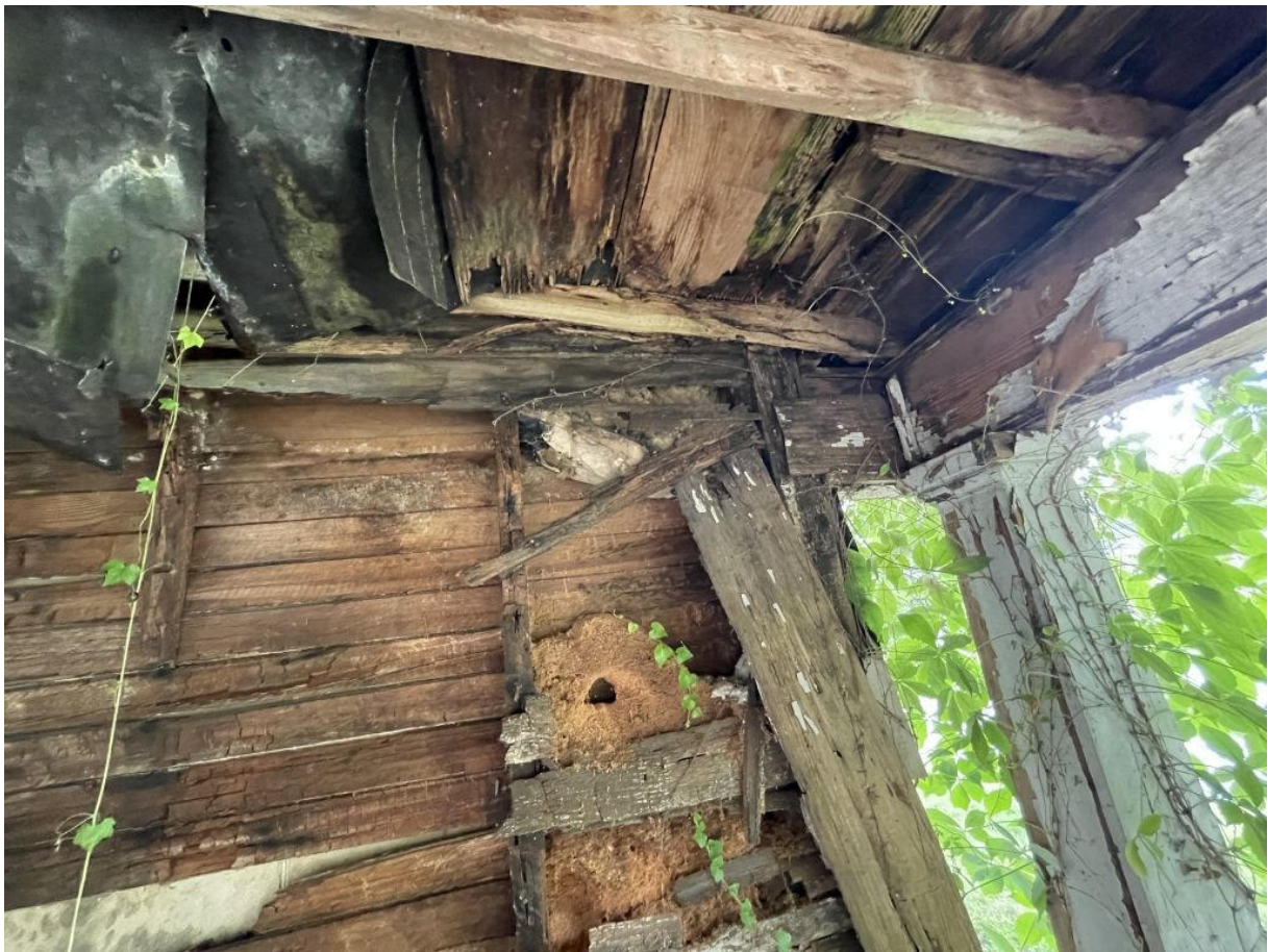
North wall of porch. Water Damage.
