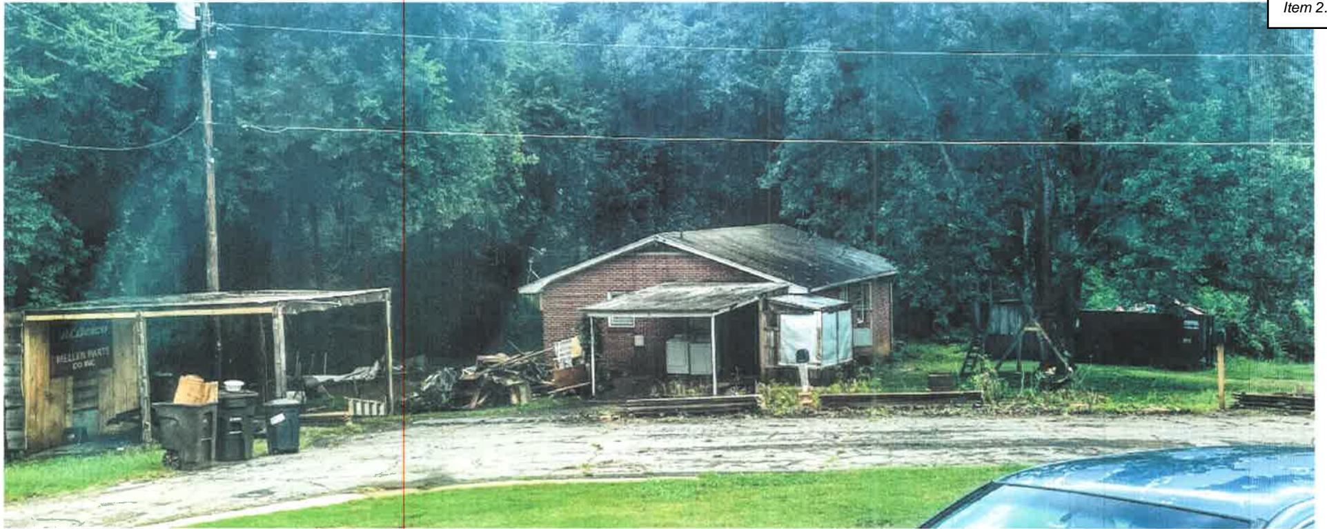
View of 7 Smith Rd. on Aug. 31 st , 2021 • newly vacant after tenants left • photo taken after start of demo (1 week in)
