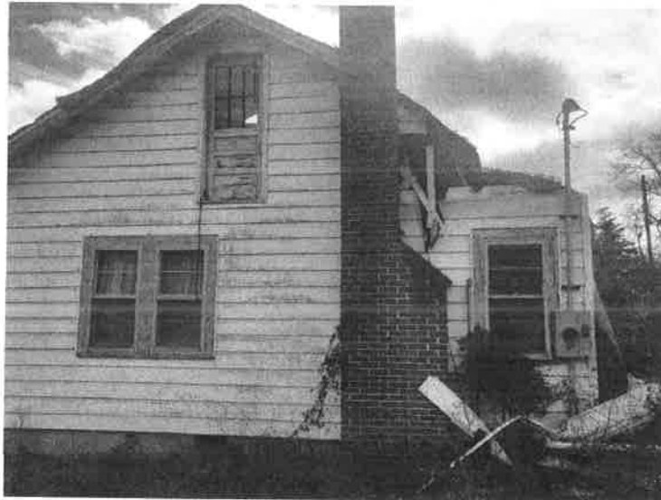
Damage to Front of the House
