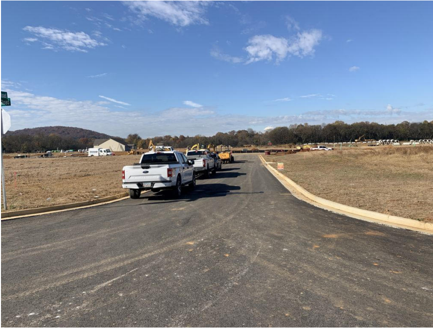
Westover Rd. at Sherwood Rd. looking West (Street lights being installed on left side)
