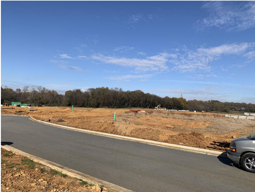
Jackson Road at Silo Rd looking Northwest toward Phase 2. (Storm pipe being installed in distance)
