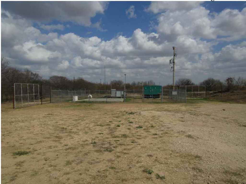
Photograph of Lift Station
