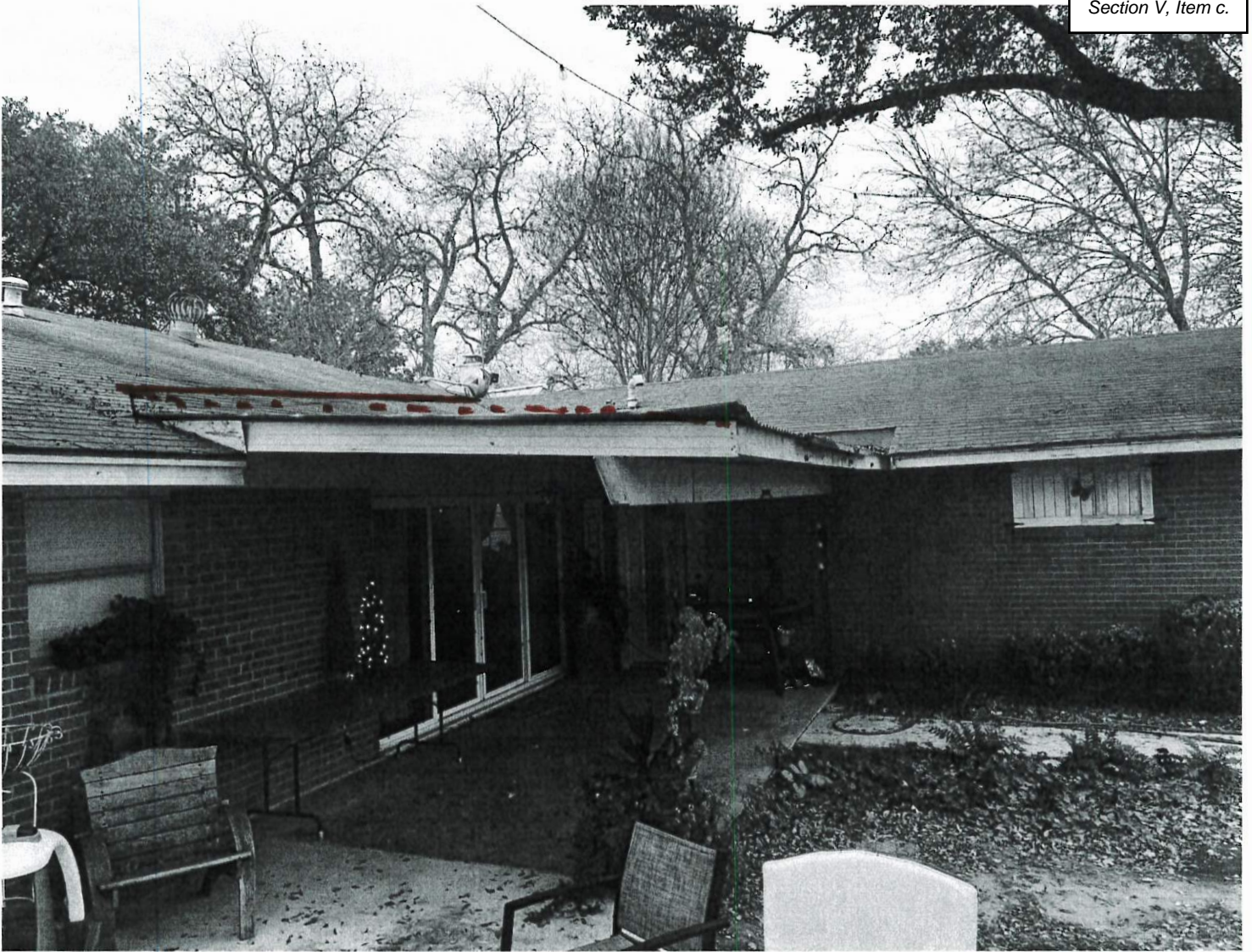
Back awning is rotting.
