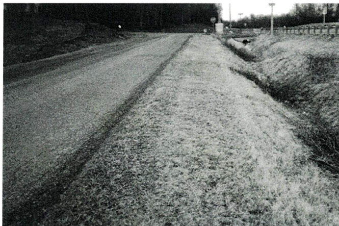
Side slope erosion can cause rollovers.
