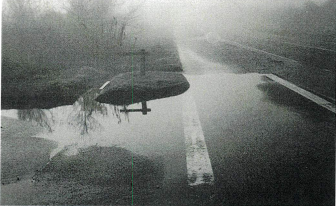
In this photo, water is ponding because the outflow ditch has silted up. Ponded water can cause drivers to leave their lane, reduce braking ability or contribute to pavement deterioration.
