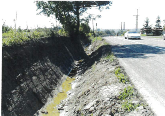
Deep ditches such as this are a safety hazard.
