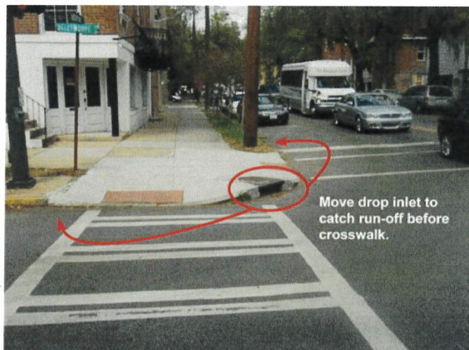
To avoid run-off across the pedestrian path, it is desirable to locate drop inlets before crosswalks.
