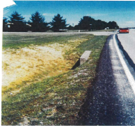
This culvert headwall is a roadside hazard.
