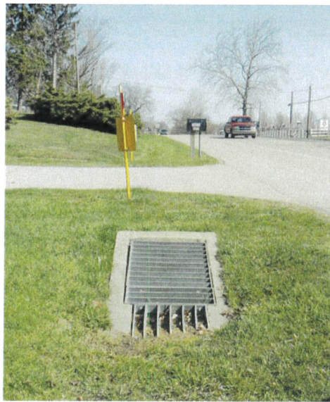
This grated inlet can be used to prevent water ponding at access points.
