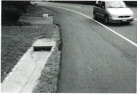
This culvert has a rather large opening which could cause a vehicle that hits it to go out of control.
