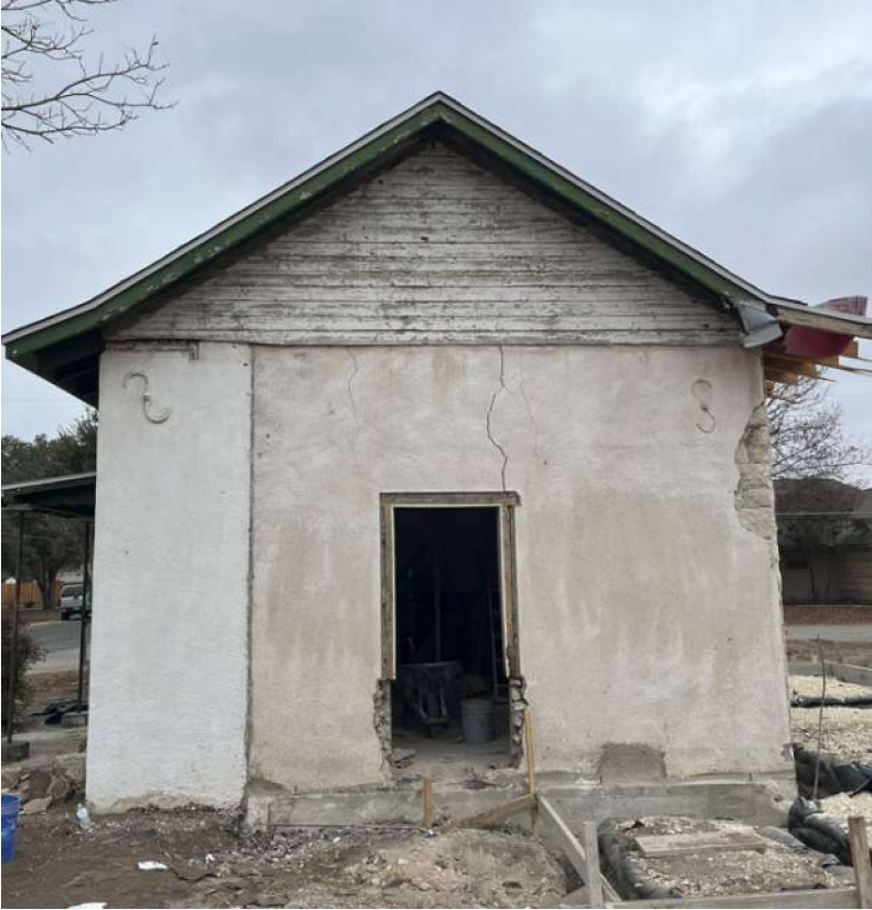
Progress photos of removing the metal lath and stucco over the original wood siding.t
