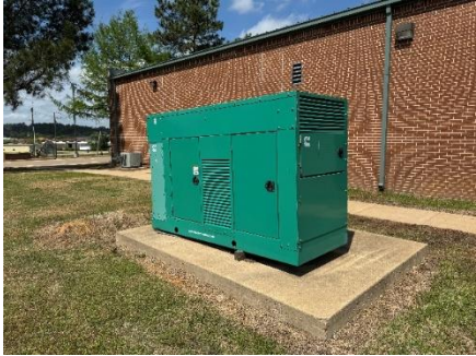
F: Natural Gas Generator
