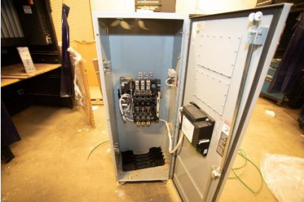
G: Electrical Transfer Switch
