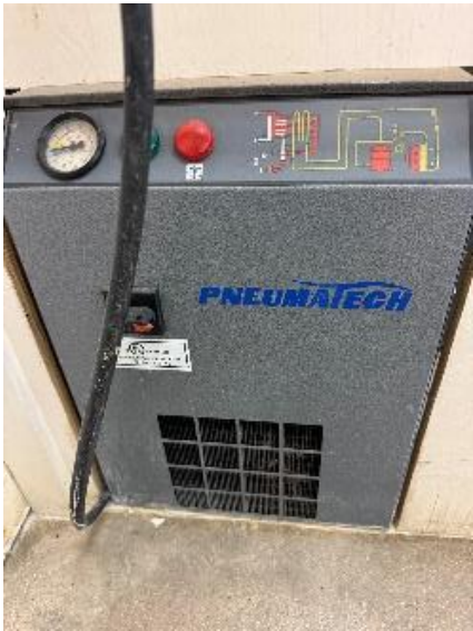
E: Compressed Air Dryer
