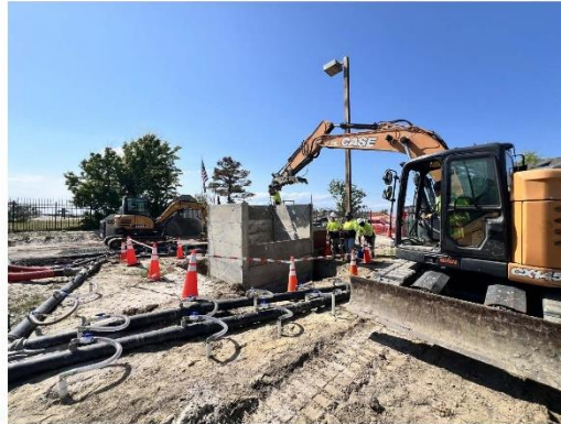
Mason Ave. Lift Station
