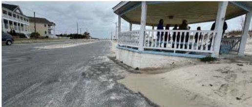
Windblown sand; the sand from the dunes is migrating past the Gazebo and into the road.
