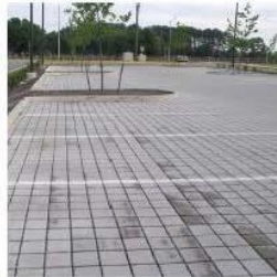
Permeable parking in parking lot
