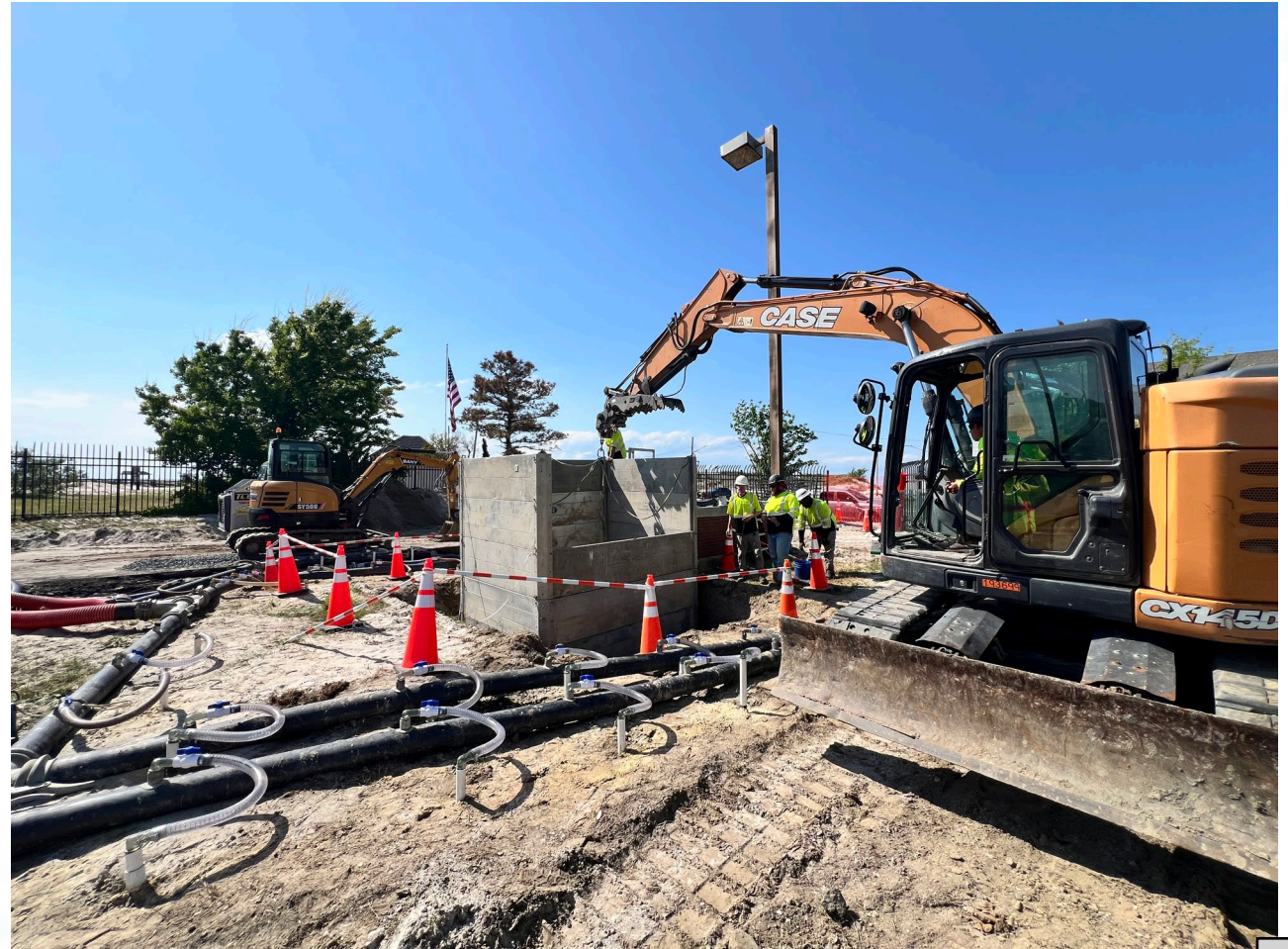
Mason Ave. Lift Station
