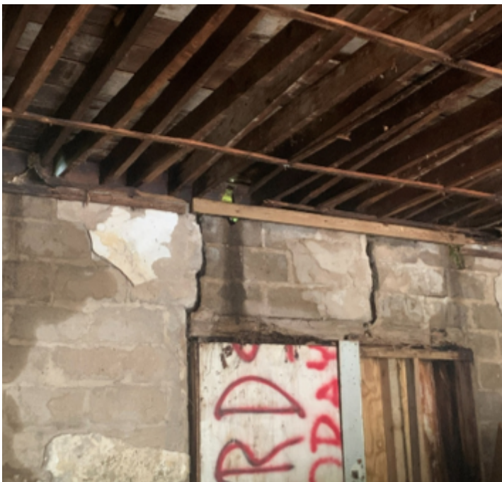
Cracking in Rear Wall
