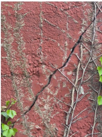
Cracking at Northwest Building Corner
