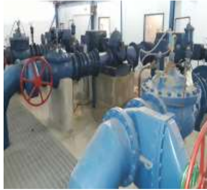
Water Loss Control Program 12% Non-revenue water loss (<15%)
