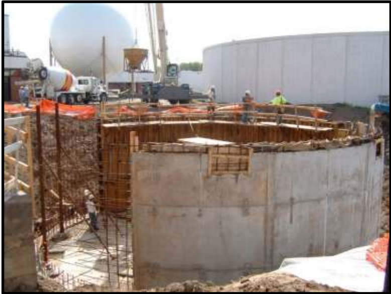
Below grade 170k gal. Receiving Tank ~2007
