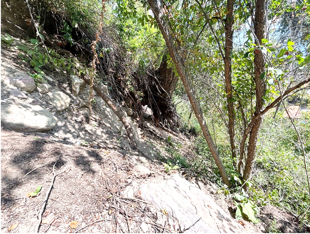
A portion of the hillside sloughing exposing boulders and undercut of tree roots
