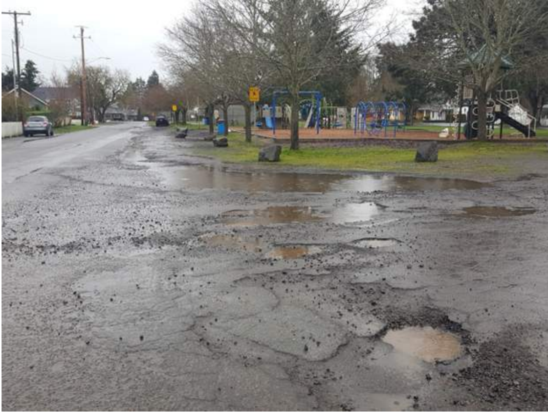
Figure 33: McKenzie and Harrison pavement and drainage condition in 2017, prior to the reconstruction project.
