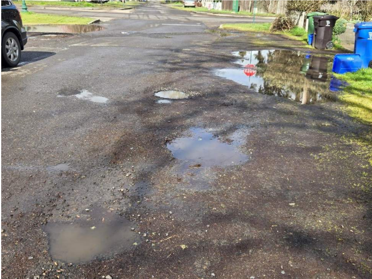
Figure 5: S. Skinner St. just south of E. Pearl St. and looking to the north, showing roadside ponding and pavement distresses.
