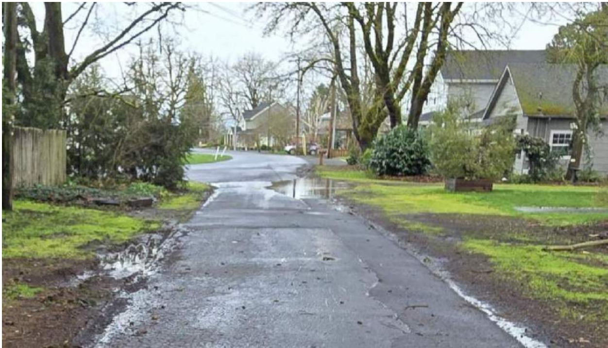
Figure 7: Ponded water on E. Locust St. due to deficient roadside infiltration, looking west to N. Diamond St.
