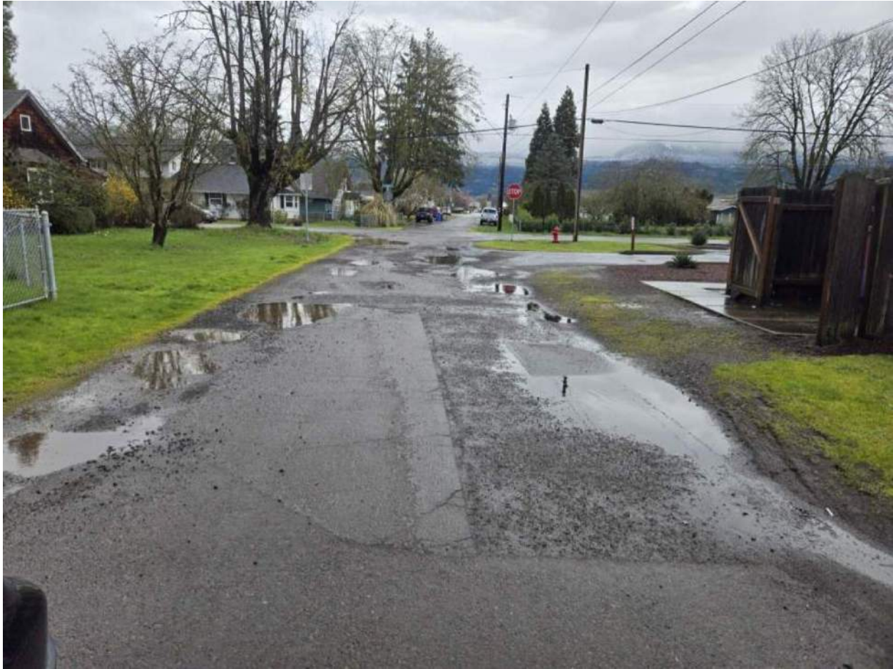
Figure 4: E. McKenzie St. between N. Coleman St. and N. Skinner St. showing degraded pavement and resulting ponded water after a mild rainfall event, looking east.
