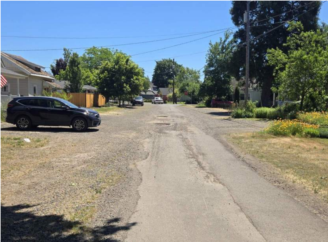
Figure 26: N. Harrison St. pavement deficiencies prior to reconstruction project in 2024.
