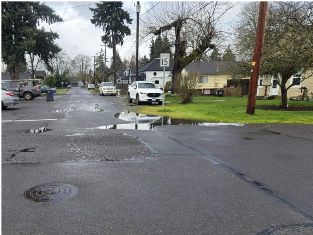
Figure 78: E. Lincoln Wy and N. Miller St. ponding, looking to the west in 2024.
