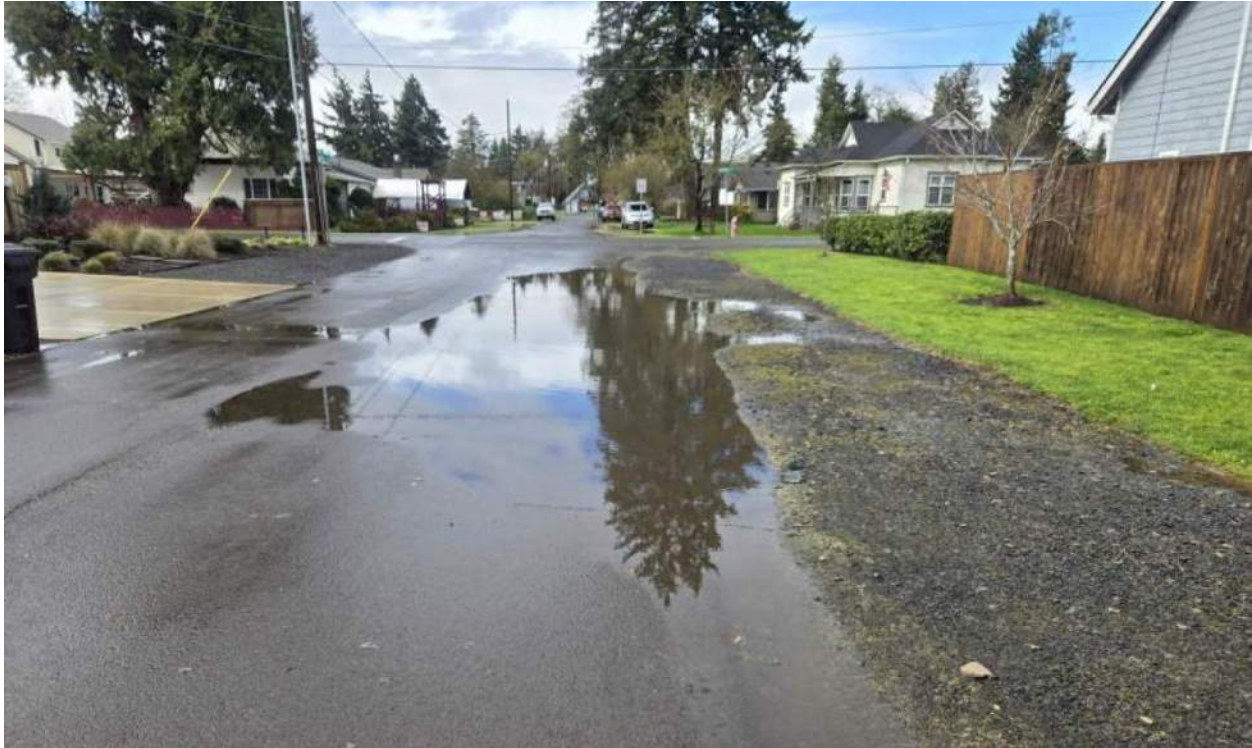
Figure 6: E. McKenzie St. looking west to N. Miller St. showing ponded water on road surfaces due to a lack of infiltration capacity in shoulder facilities.
