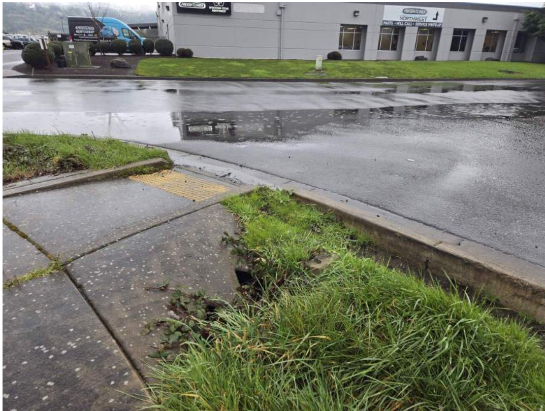
Figure 92: Coburg Industrial Way overgrown culvert in 2024.
