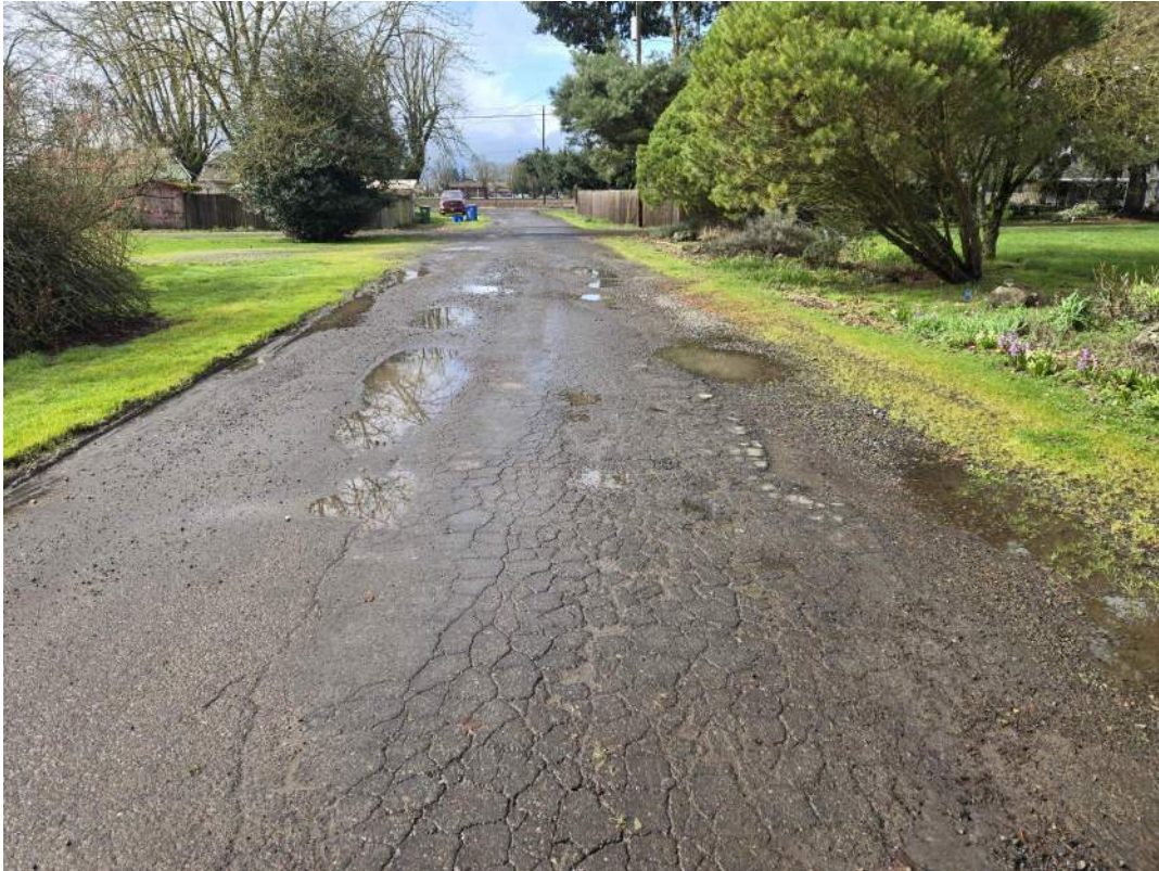
Figure 27: E. Macy St. pavement deficiencies prior to reconstruction project in 2024.
