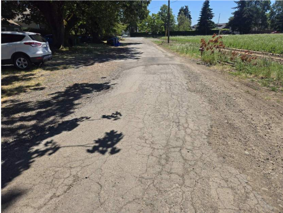
Figure 28: N. Willamette St. pavement deficiencies prior to reconstruction project in 2024.
