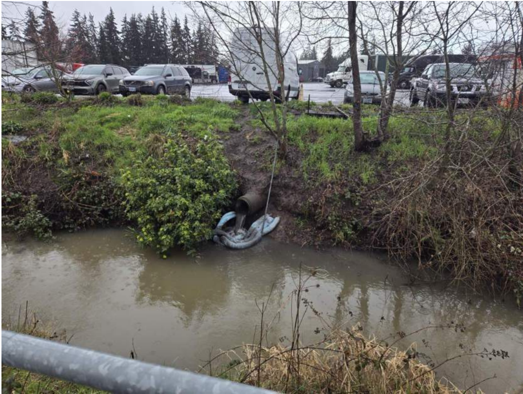
Figure 21: Coburg Travel Center of America outfall to Muddy Creek along Coburg Industrial Way in 2024.
