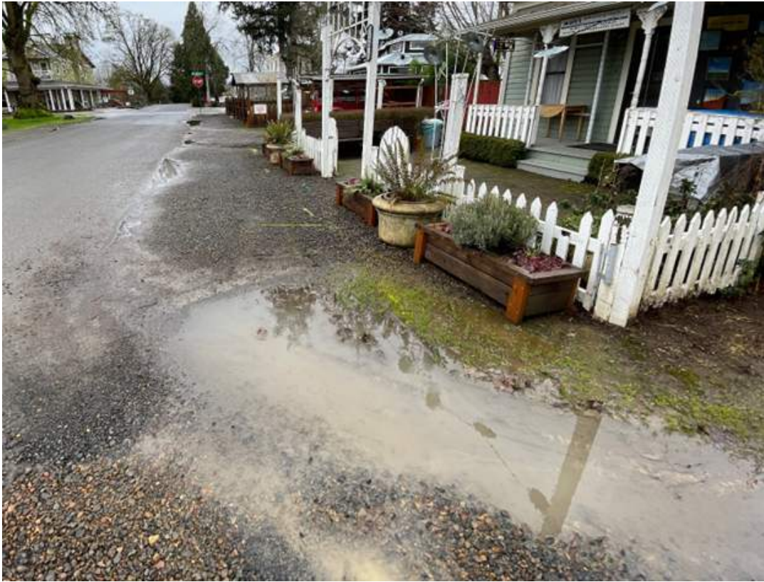
Figure 37: McKenzie St. drainage condition in 2021 prior to the 2022 reconstruction project.
