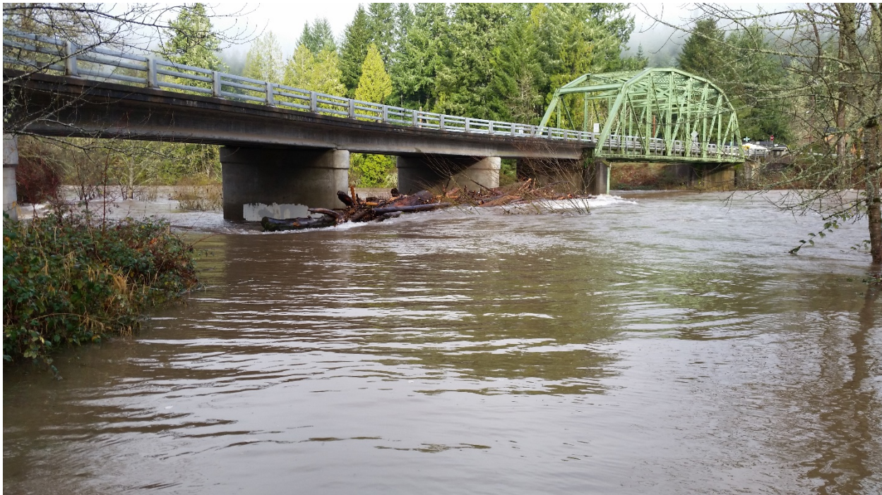
Bridge Street bridge experiencing rising waters and debris during a December 2014 event. | Photo: Lane County Public Works, Roads Division
