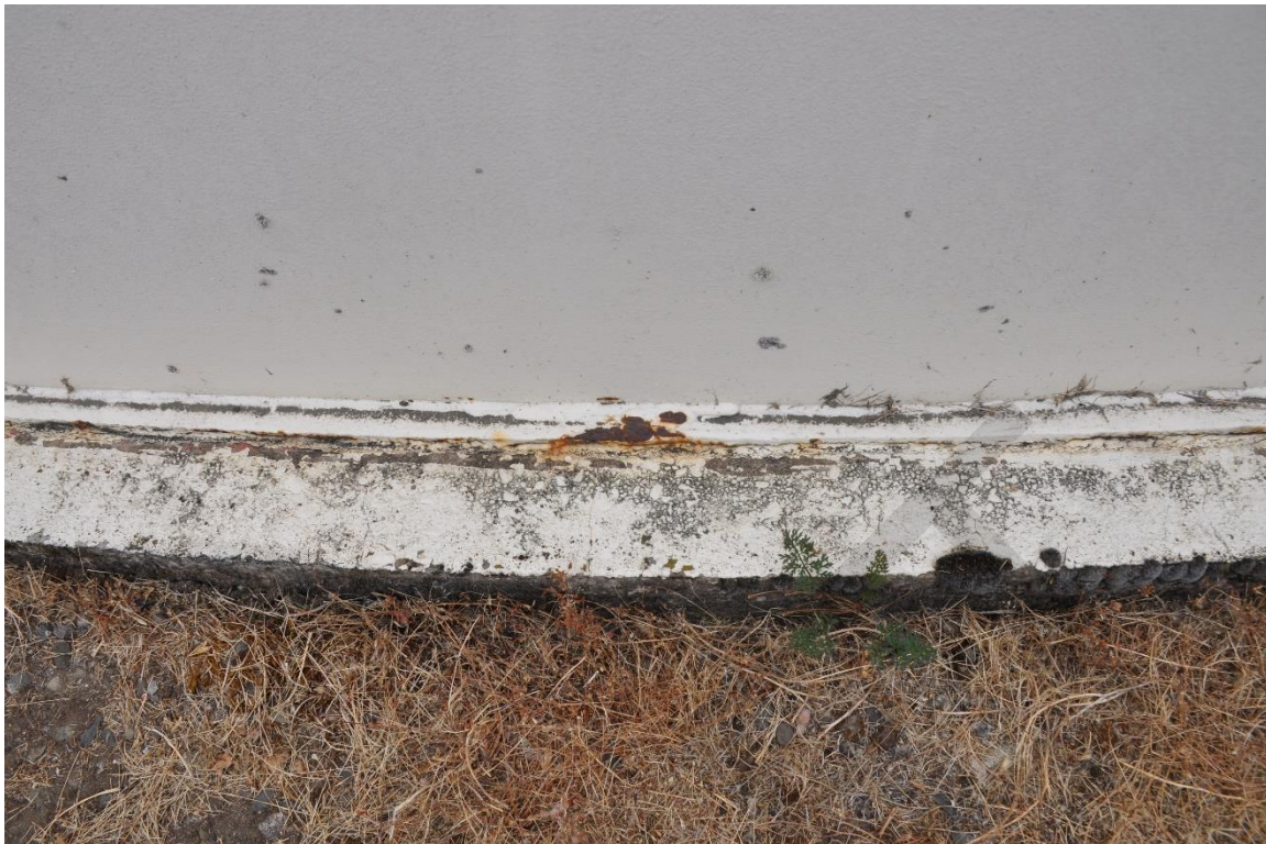
Photo 20 – Tank Exterior Coating Deterioration
