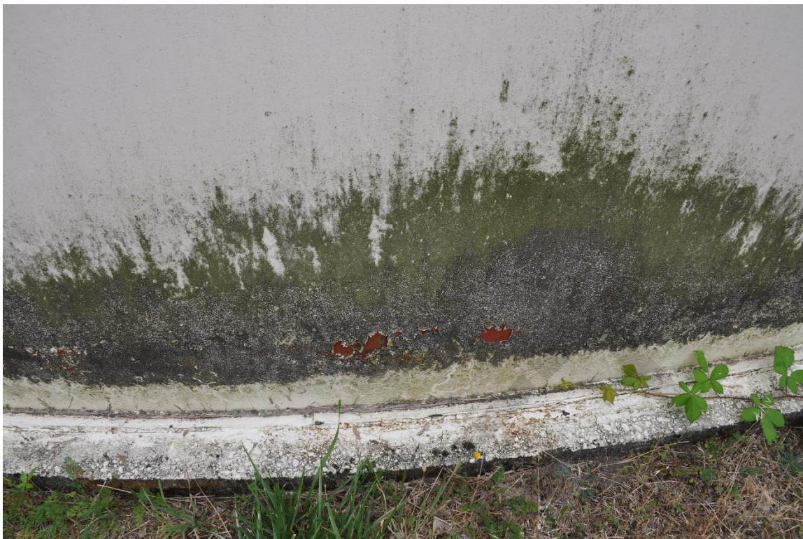
Photo 7 – Tank Exterior Coating Deterioration
