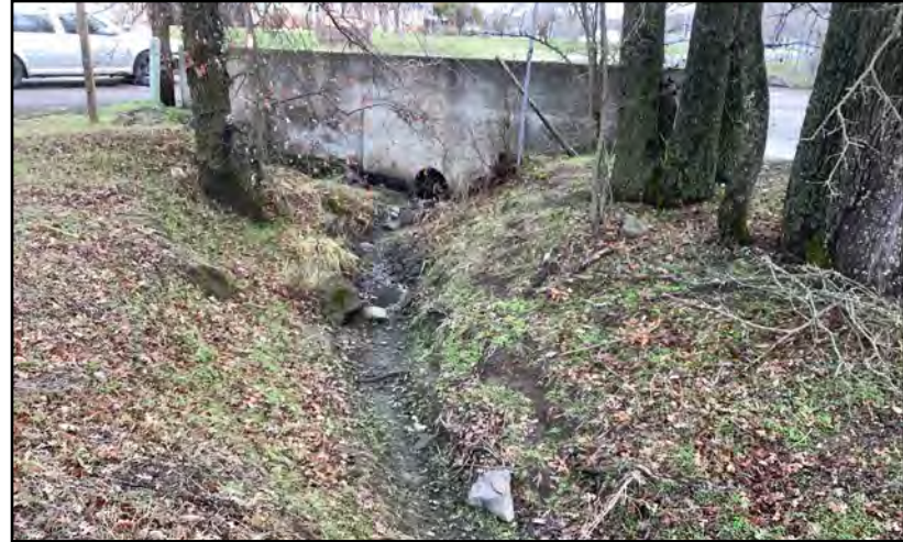
Photo 2. Culverted inlet for the onsite drainage located in the northeast corner of the Study Area. Photo taken January 29, 2021, facing west.
