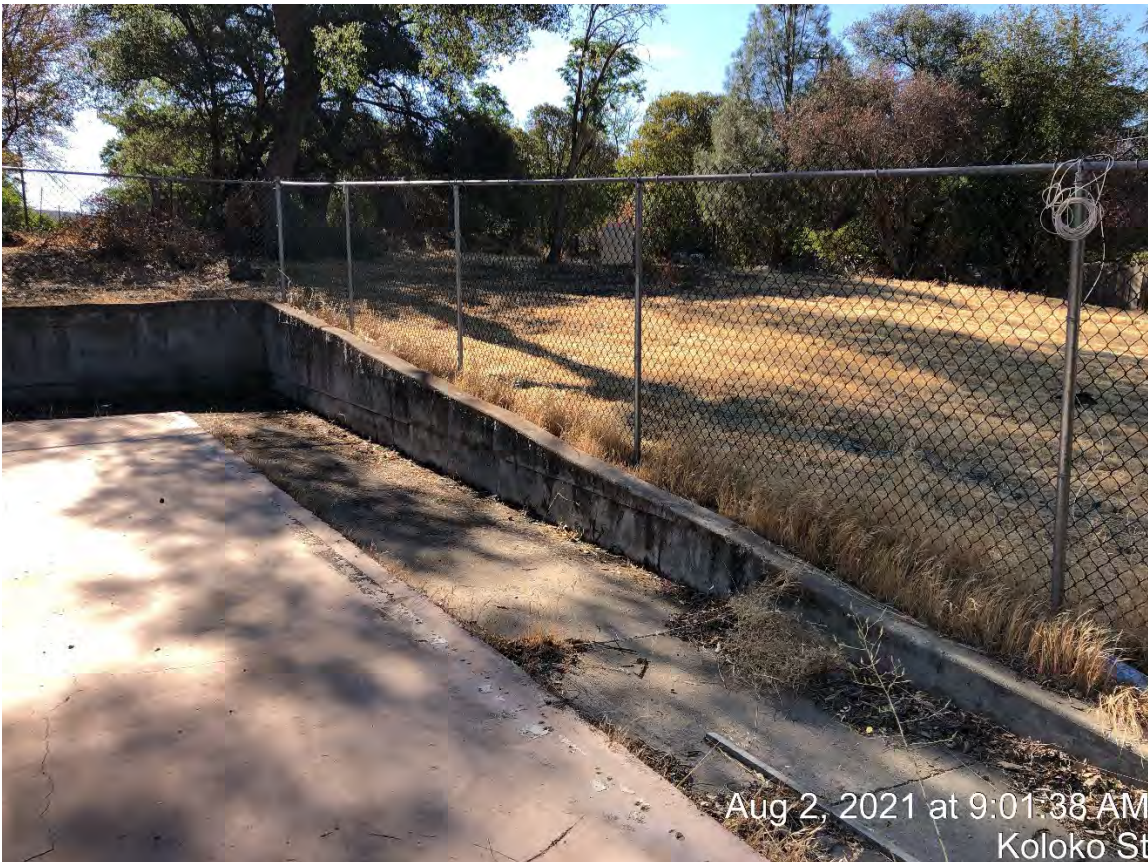
View 18: Looking southeasterly, towards high grade on project site. Existing building slab in foreground.
