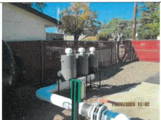
Photo 18: A photo of the carbon odor control system at Pump Station No. 3.
