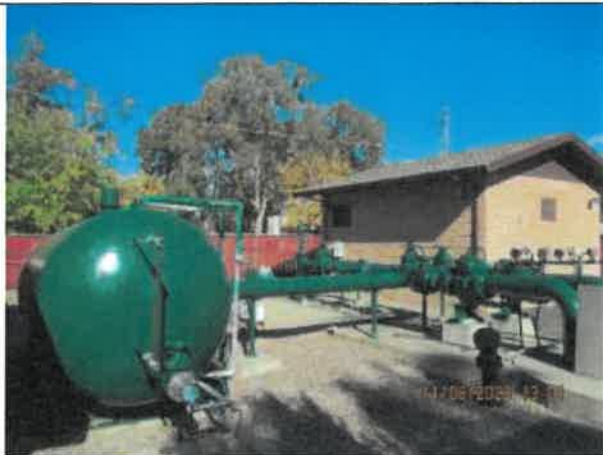
Photo 19: A photo of the recently painted aboveground pumps and piping system at Pump Station No. 3.
