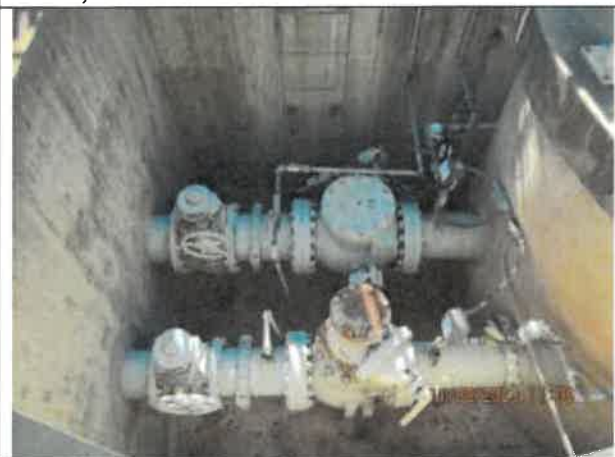
Photo 5: A photo of the one of the uncovered dry wells with minimal debris and paint chippings.
