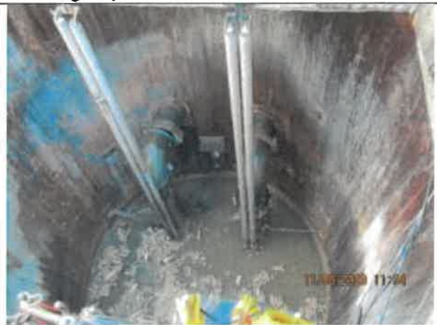
Photo 12: A photo of the south wet well at Pump Station No. 2 showing minor debris, FOG, and staining on the walls. The disconnected pipe in the photo is currently under repairs.
