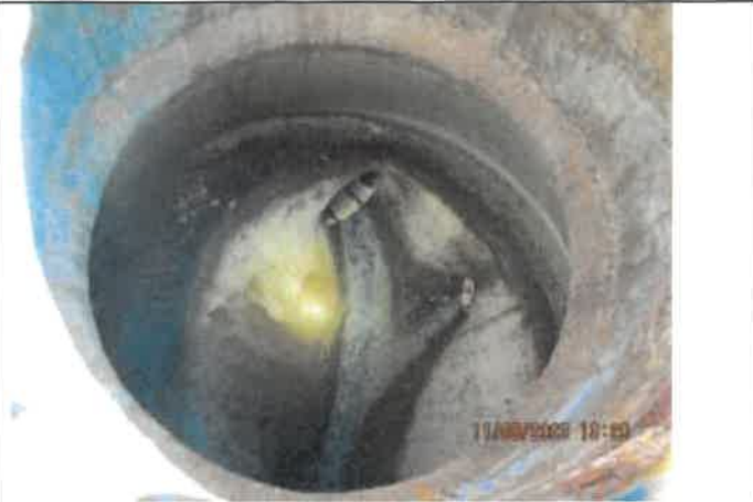
Photo 24: A photo on the manhole located in front of 6825 Meadowbrook Drive low flow and FOG on the sides of the manhole channel.
