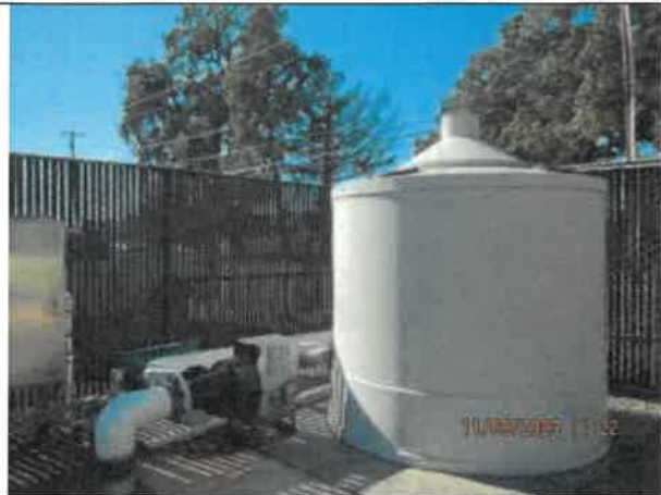
Photo 8: A photo of the carbon filter system at Pump Station No. 1 for odor control.
