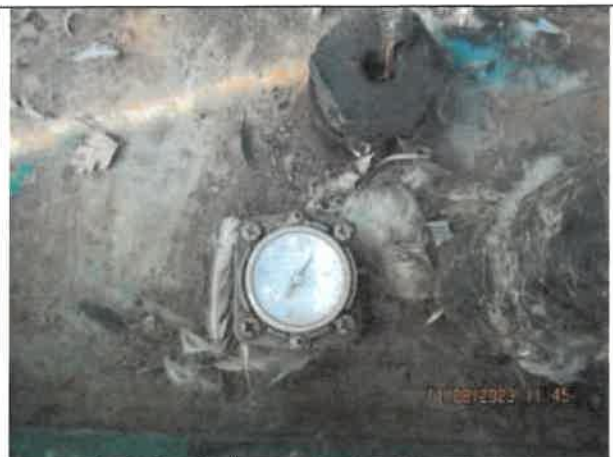
Photo 16: A photo of the fuel level of the generator at Pump Station No. 2 showing the fuel level to be over half full.
