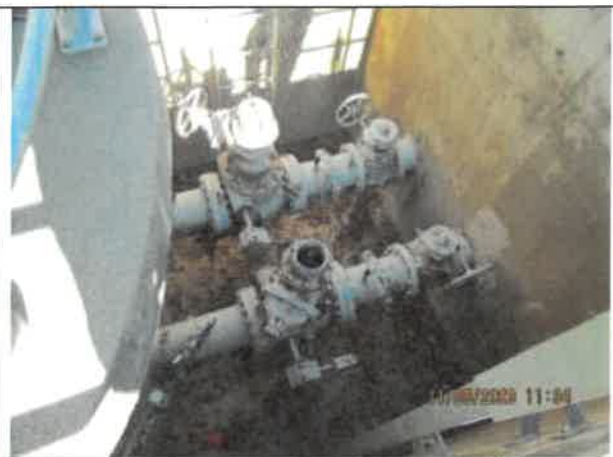
Photo 10: A photo of the uncovered south dry well at Pump Station No. 2 showing debris and a missing cap on one of the connections.
