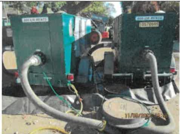
Photo 29: A photo of the portable bypass system being used while Pump Station No. 6 is under construction.
