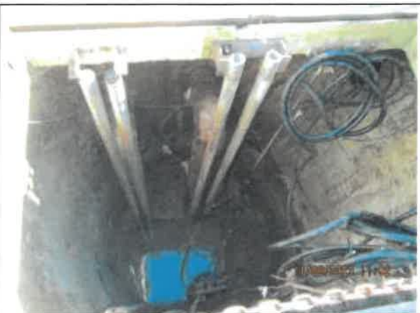
Photo 2: A photo of the wet well on the south side of Pump Station No. 1 with minor FOG, rags, and corrosion.
