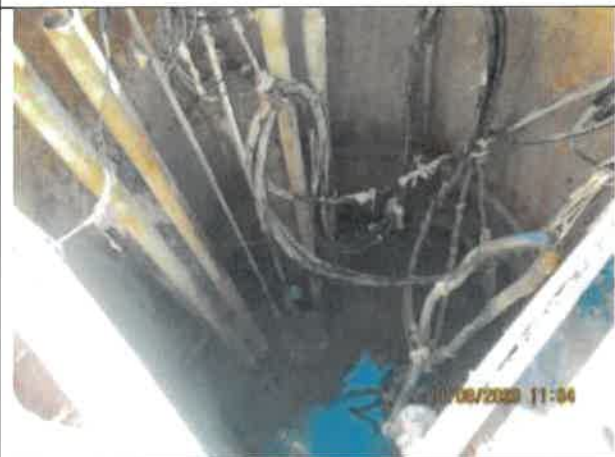
Photo 3: A photo of the wet well on the north side of Pump Station No. 1 with rags, minor FOG, and minor corrosion.
