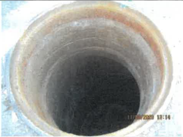
Photo 22: A photo on the manhole located at the intersection of Bay Street and Lakeview Way with corrosion around the rim and staining in the barrel.
