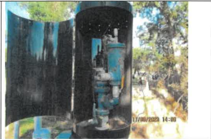
Photo 31: A photo of the ARV located at the aerial crossing with cobwebs around the ARV.
