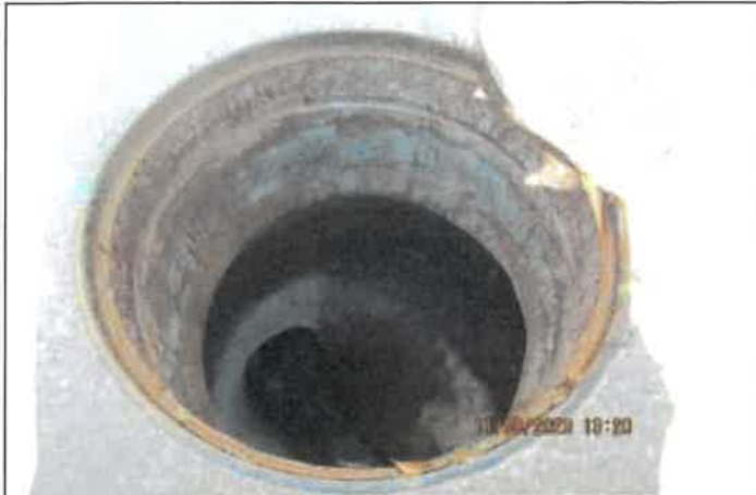
Photo 23: A photo on the manhole located in front of 6825 Meadowbrook Drive with corrosion around the rim.
