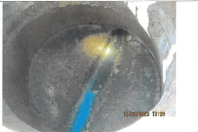
Photo 26: A photo on the manhole located in front of 6925 Meadowbrook Drive with a vertical crack in the manhole barrier and no flow in the channel.
