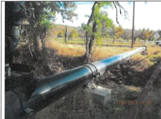
Photo 30: A photo of the force main aerial crossing located at the intersection of Rusmey Road and Pamela Lane with no secondary encasement.
