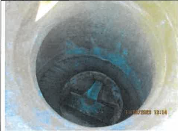
Photo 21: A photo on the manhole located at the intersection of Bay Street and Lakeview Way with fast flow.
