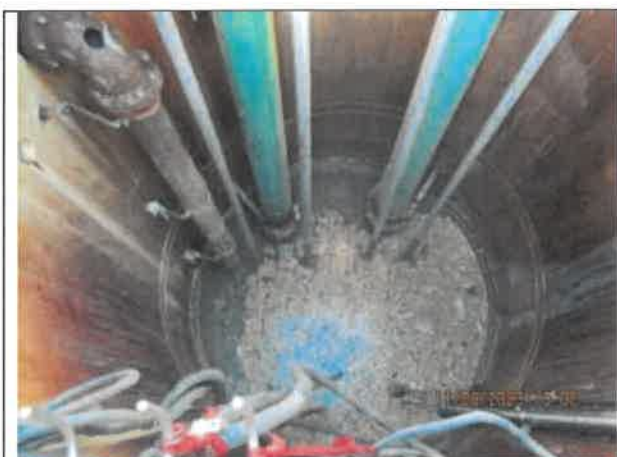
Photo 17: A photo of the wet well at Pump Station No. 3 showing a FOG mat, rags on the pipes, corrosion, and staining on the walls.
