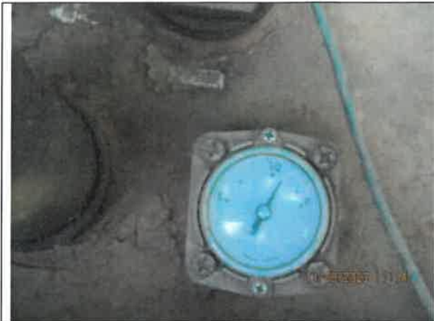
Photo 7: A photo of the fuel level of the generator at Pump Station No. 1 showing over 50 percent full.
