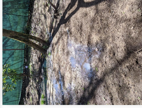
Property in 2021 Effluent surfacing from failing septic system
