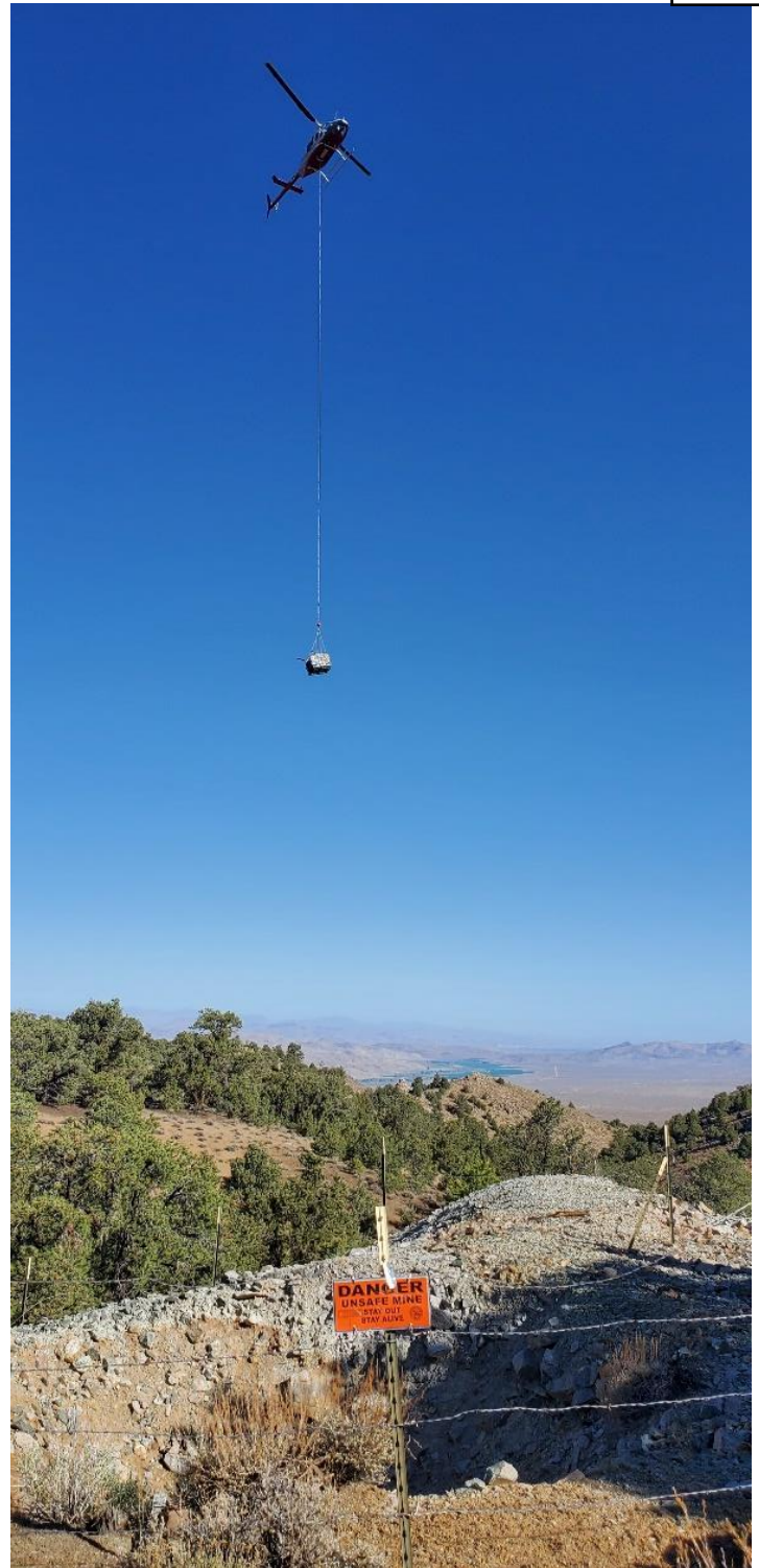
Picture 4 – Helicopter sling line aided delivery of closure supplies at WRSP permanent closure project, Lyon County, Nev.
