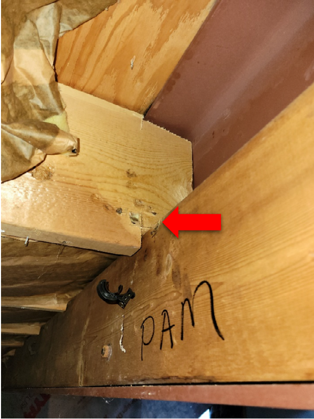
Notched Joist at Steel Beam
