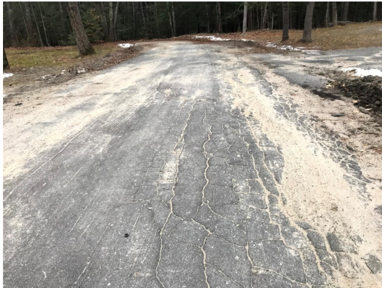
Rutting – Ring Landing Road
