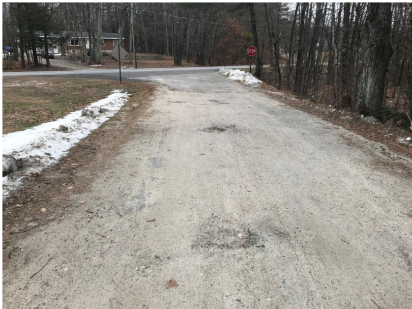
Potholes – Varney Road
