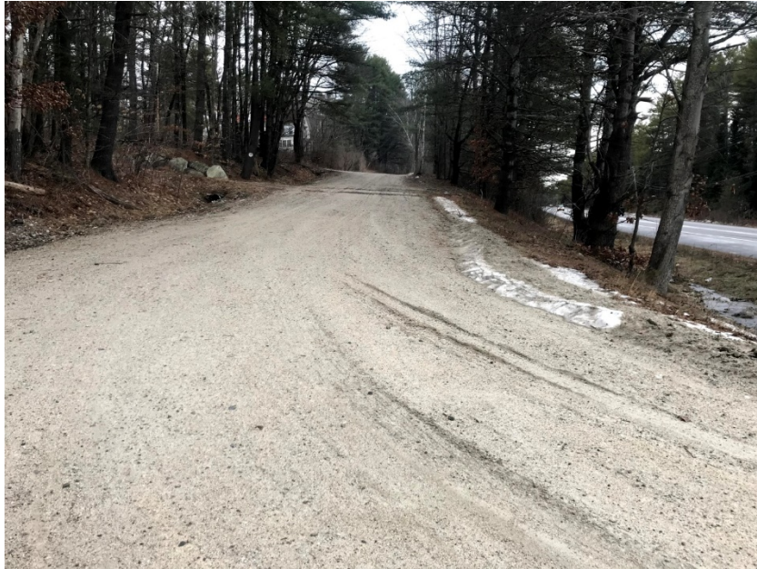
Rutting – Bramble Hill Road
