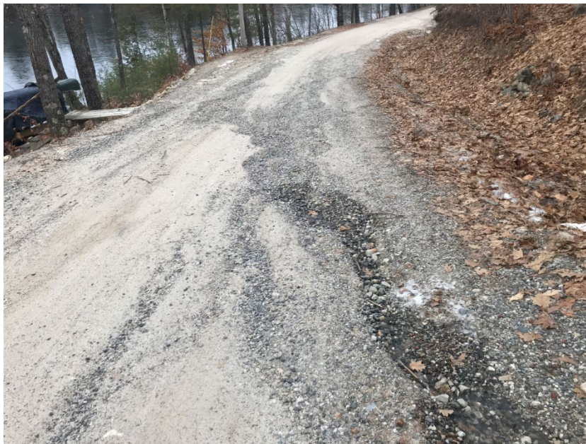
Loose Aggregate – Lord Road
