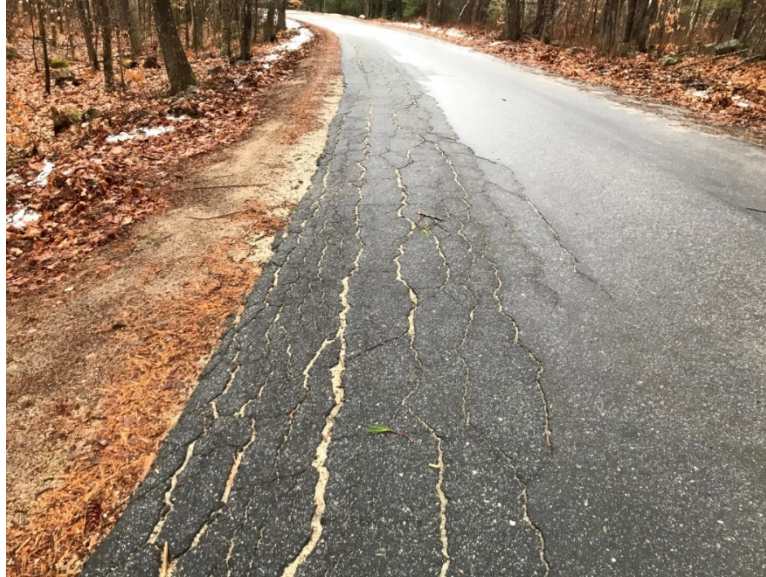
Edge Cracking – Jim Small Road
