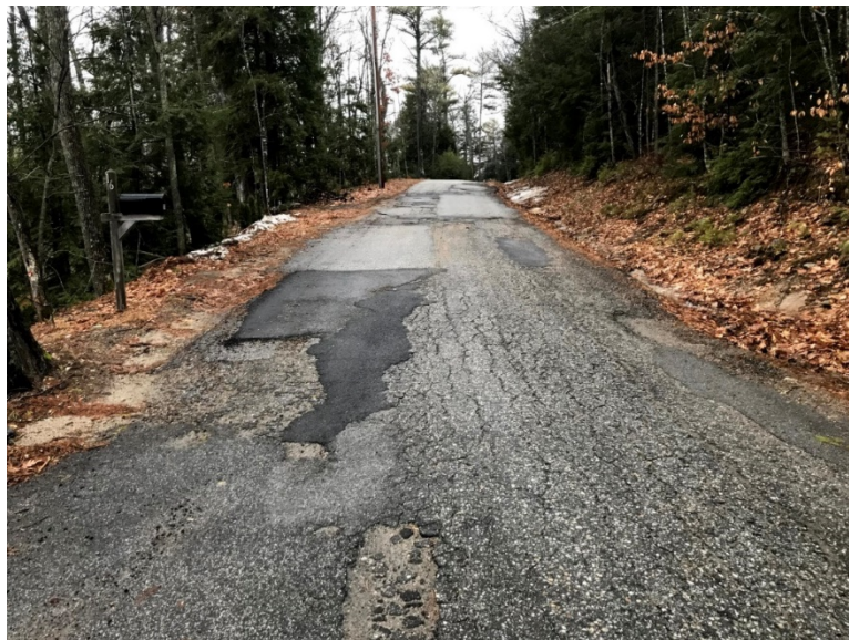
Patching/Potholes – Stone Road
