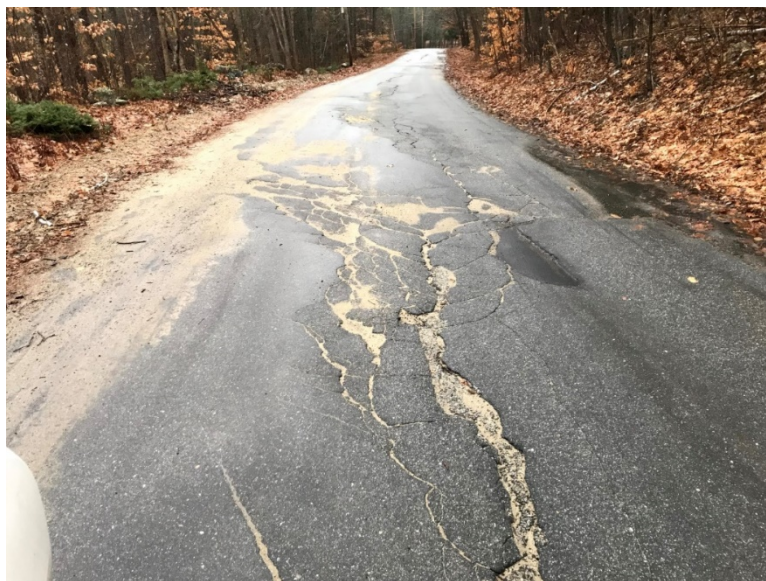
Longitudinal Cracking – Burgess Road
