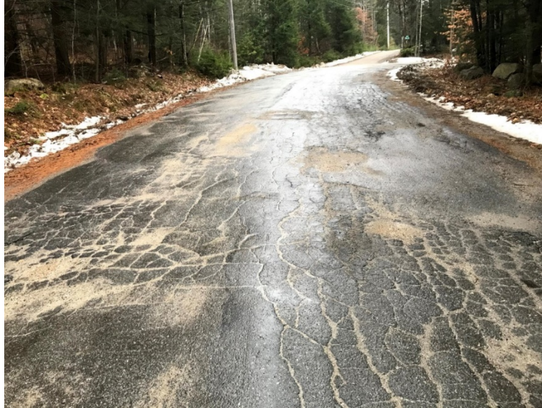
Alligator Cracking – New Road
