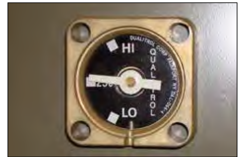
Figure 5. Liquid level gauge.
