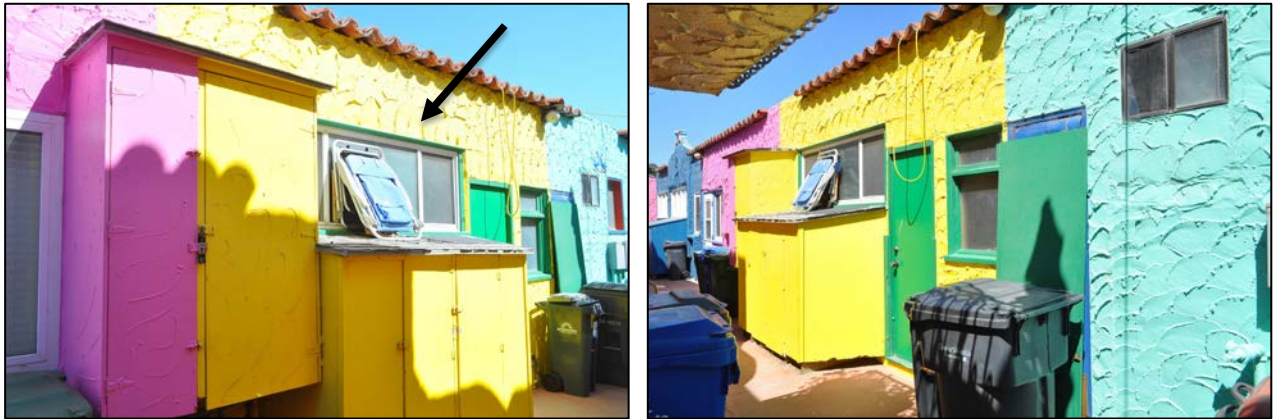
Figures 3 and 4. Two images of the rear (north) elevation, as viewed from the alley. The horizontal window (arrow) is not original to the building.
