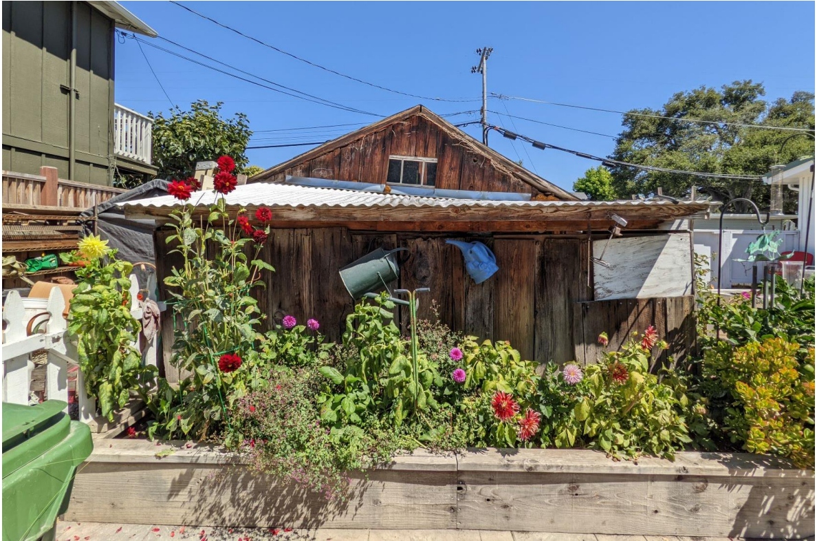
Rear of Detached Garage and Shed Addition – 529 Capitola Ave., Viewed from the south, August 2022 (Photo by Leslie Dill)
