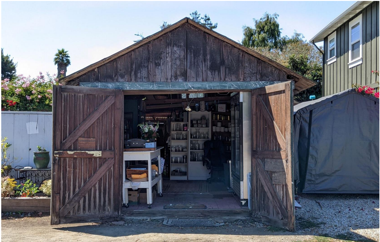
Detached Garage – 529 Capitola Ave., Viewed from the north (from Beverly Avenue), August 2022 (Photo by Leslie Dill)
