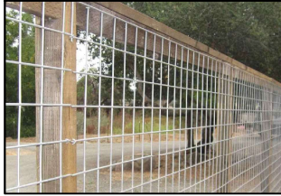
NEW PERIMETER FENCE: 6' TALL WELDED WIRE MESH PANEL WOOD MEMBERS: STAIN PLATINUM GRAY
