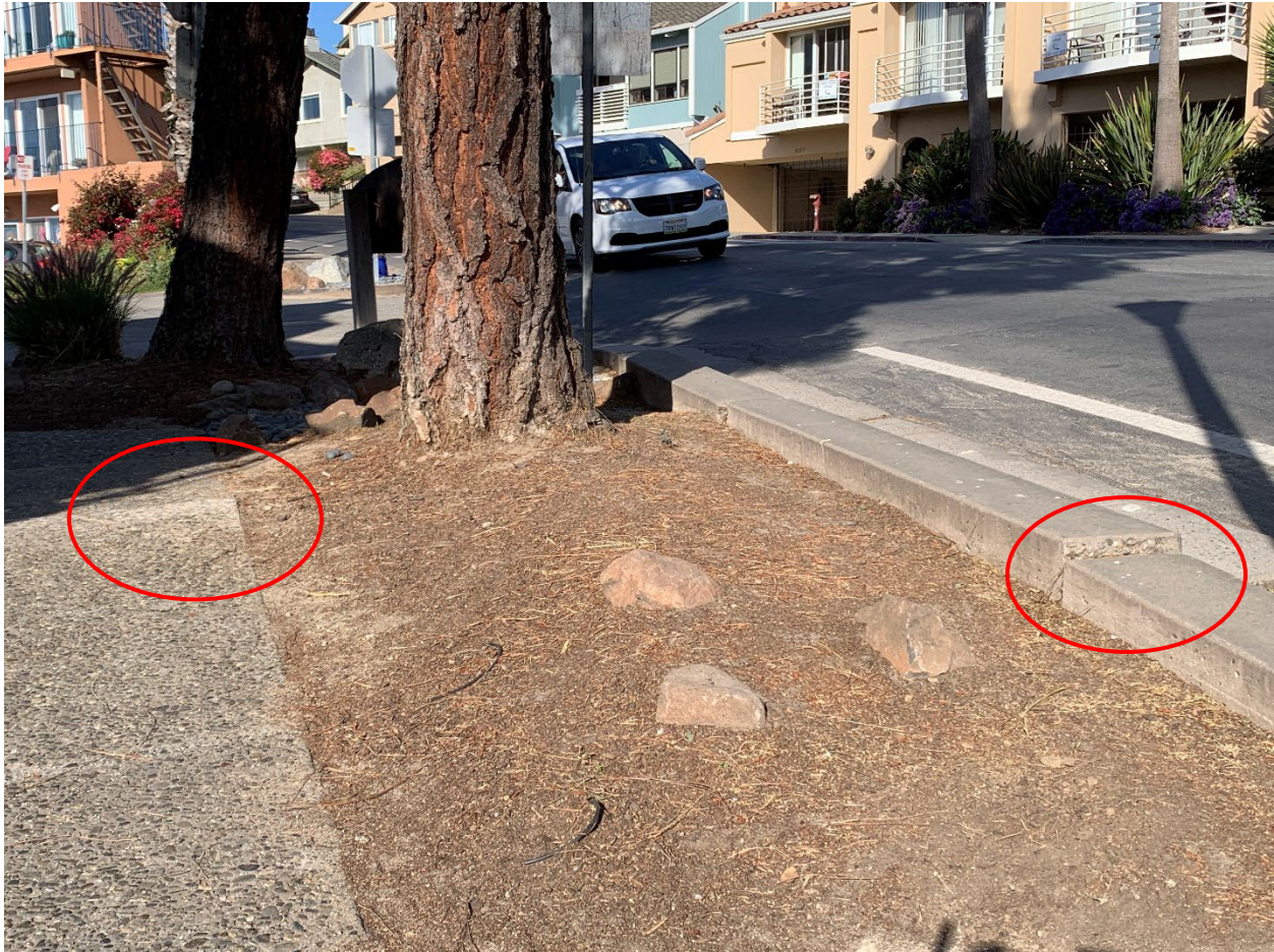
Image #6 – Tree T2 sidewalk damage and lifted curb.
