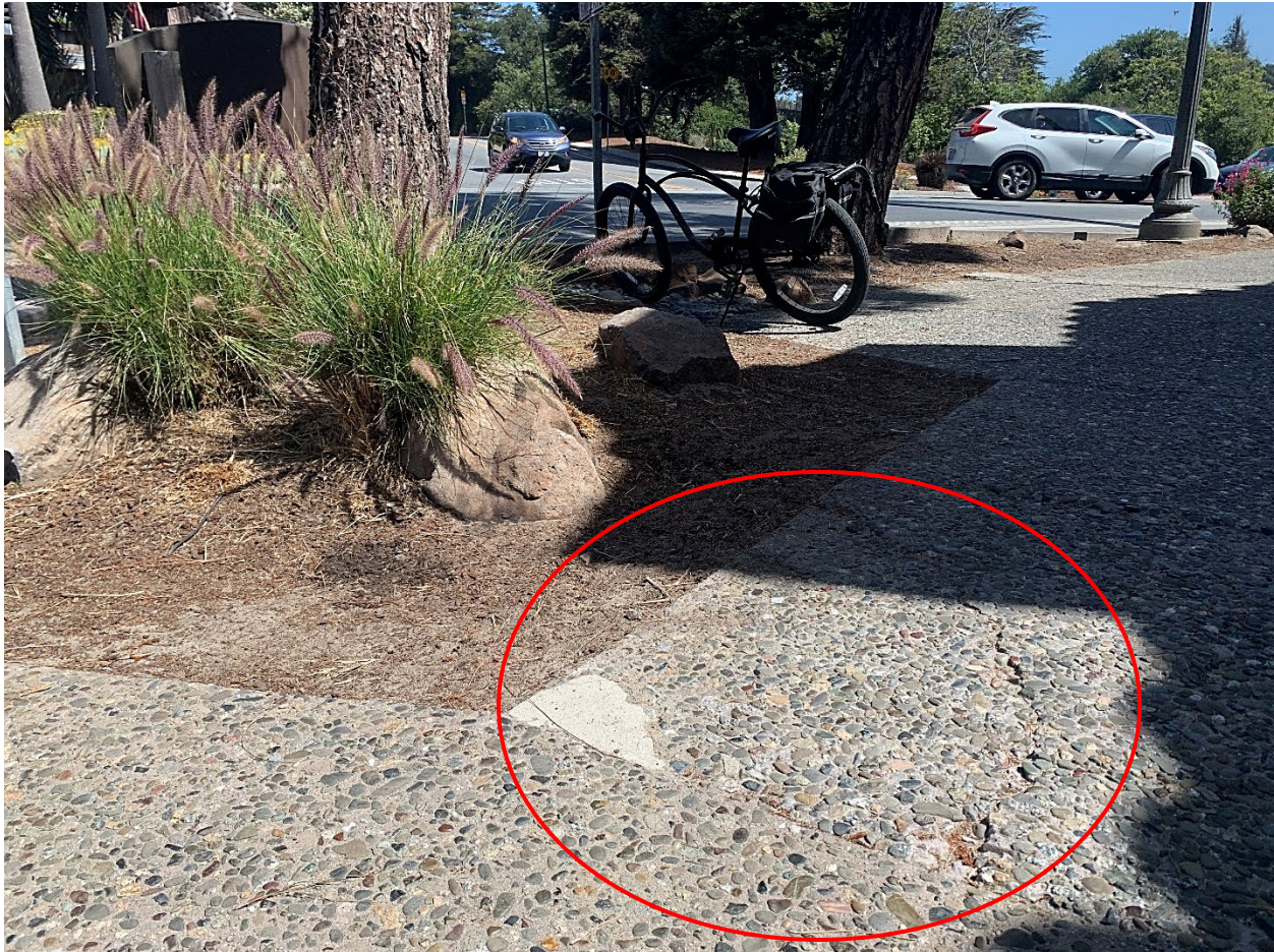
Image #7 – Sidewalk damage from tree T1. Note corner of sidewalk has been repaired
