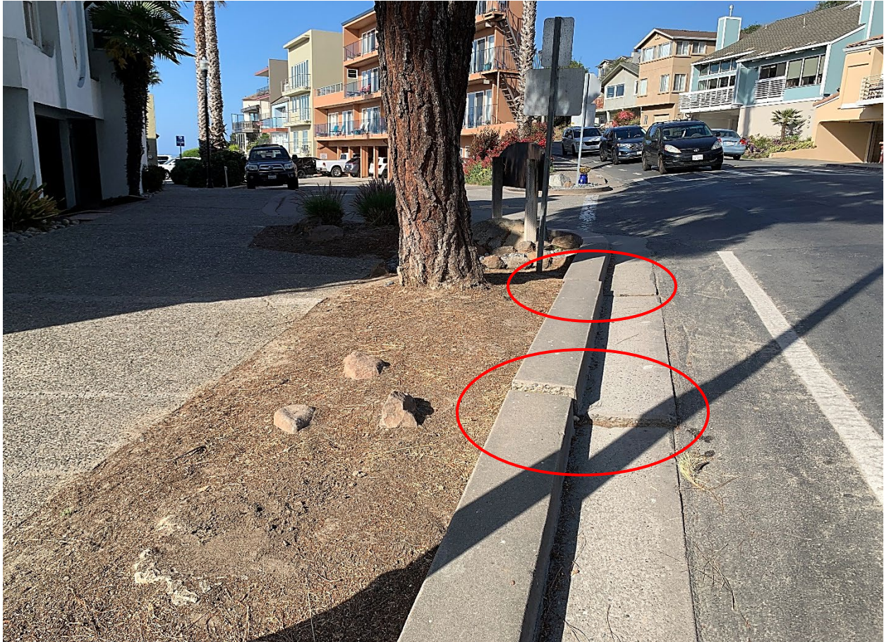
Image #5 – Curb and gutter damage from tree T2., (circled). The asphalt connected to the gutter is also showing damage.
