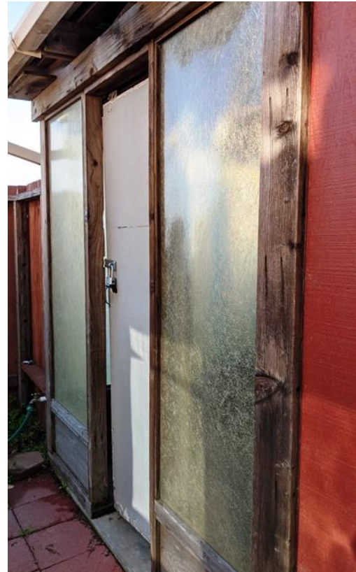
North Entrance to Greenhouse. Viewed facing east. January 2020. (Photo by Leslie Dill)
