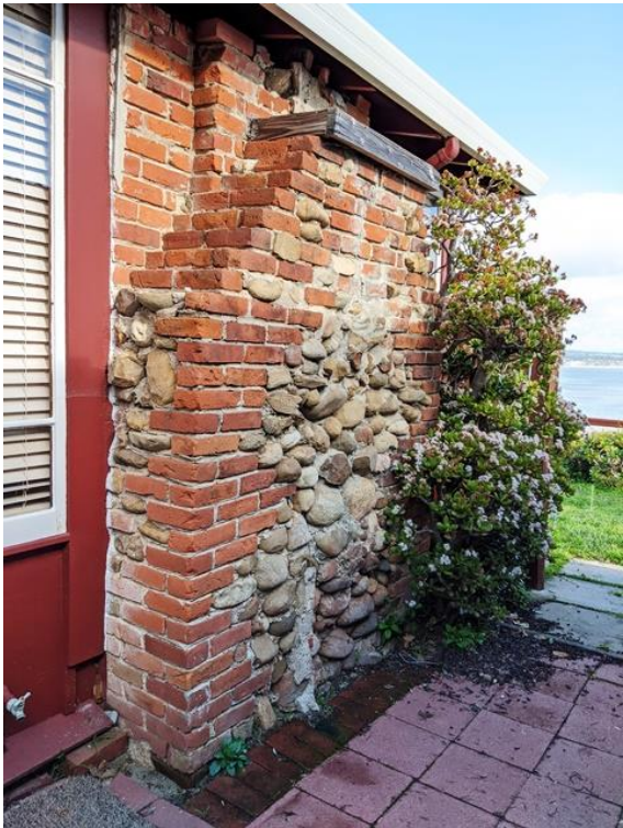
Detail of Chimney at South Façade. Viewed facing northeast. January 2020. (Photo by Leslie Dill)
