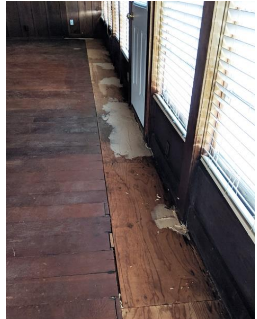
Detail of Living Room Floor Repair. Viewed facing north. January 2020. (Photo by Leslie Dill)
