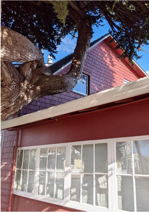
South Elevation. Showing upstairs windows and enclosed former front porch. Viewed facing northeast. January 2020. (Photo by Leslie Dill)
