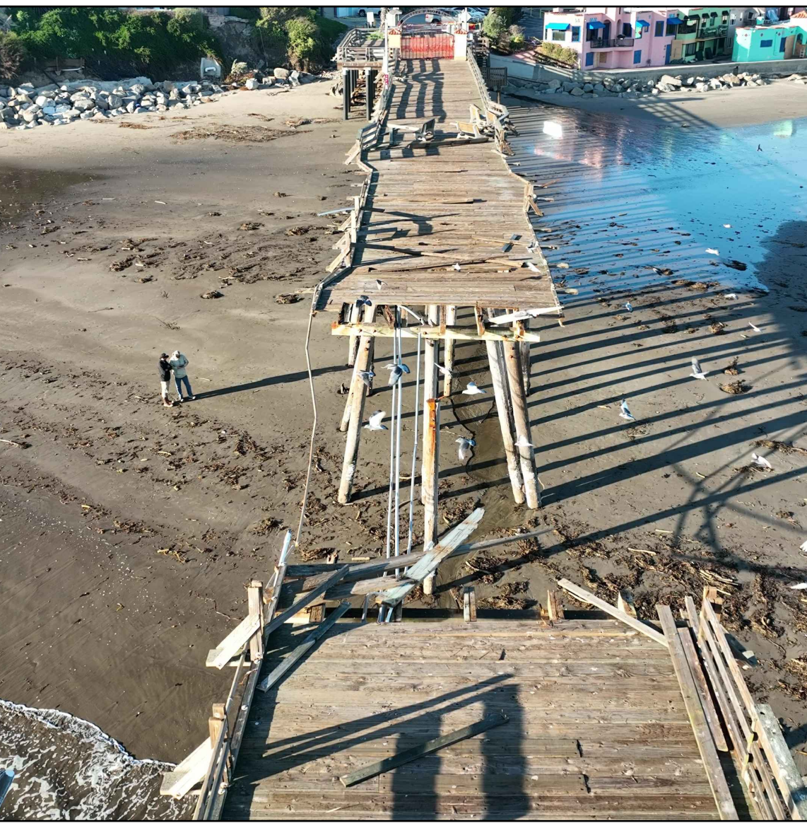
PHOTO 11 STORM DAMAGE AT TRESTLE
