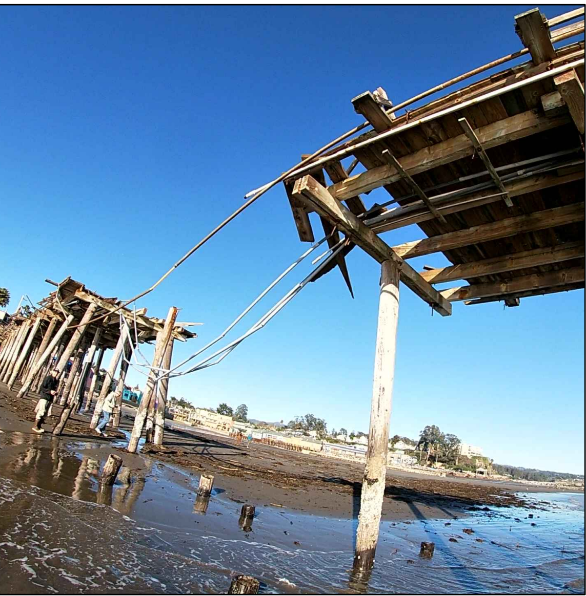
PHOTO 12 STORM DAMAGE AT TRESTLE
