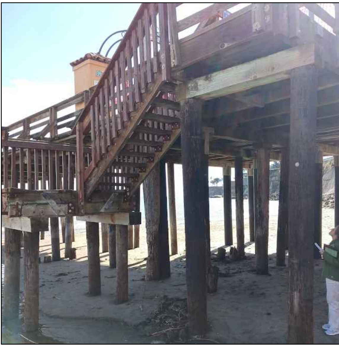
PHOTO 9 STORM DAMAGE AT STAIRS
