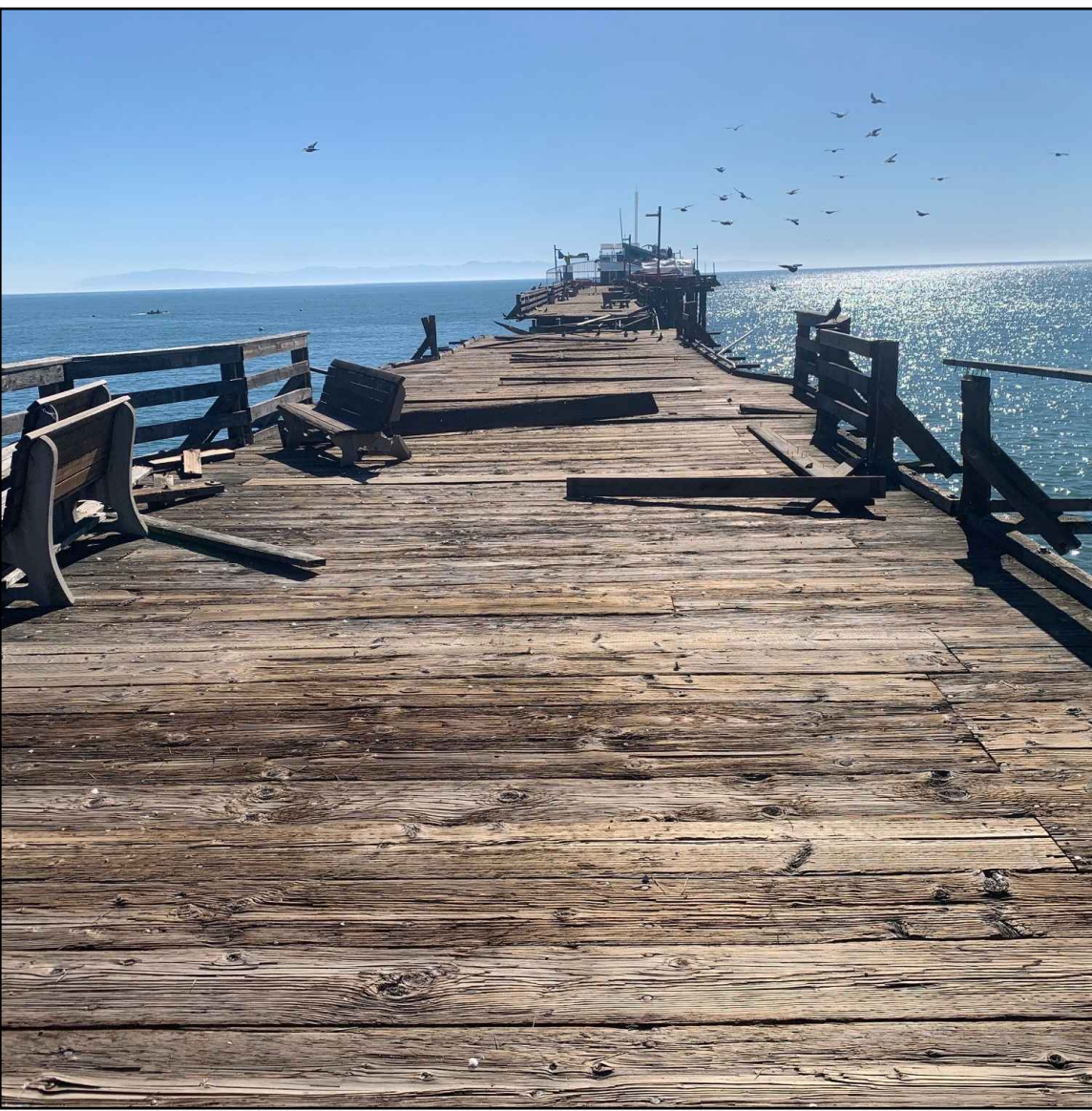
PHOTO 10 STORM DAMAGE AT TRESTLE
