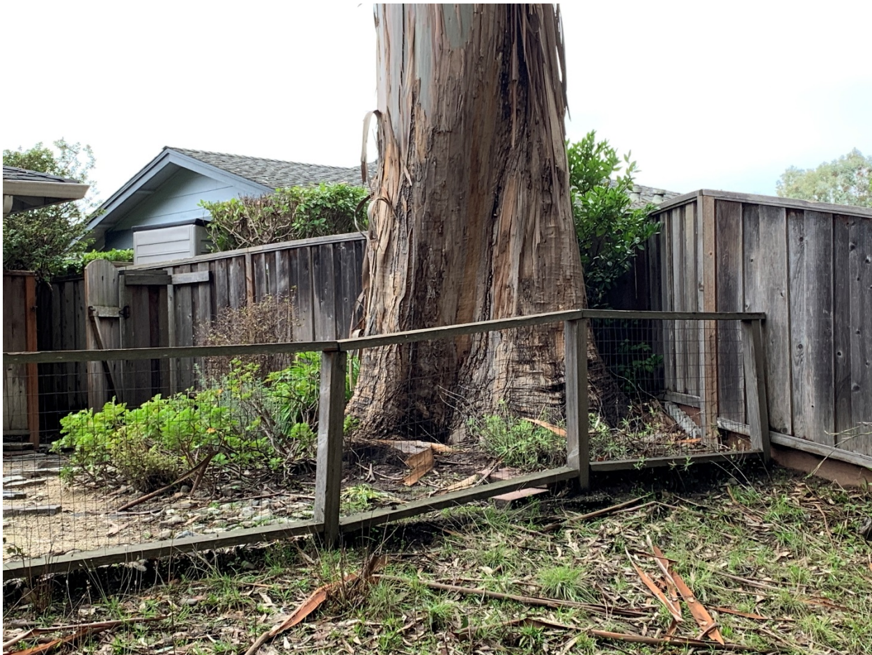
Image #2 – Well tapered trunk. Location is on fence line at top of slope with good rooting area below.
