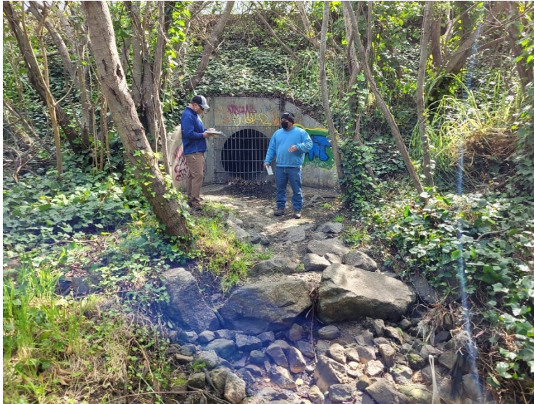
Figure 9. Simpkins Ditch and Outfall with Trash Rack
