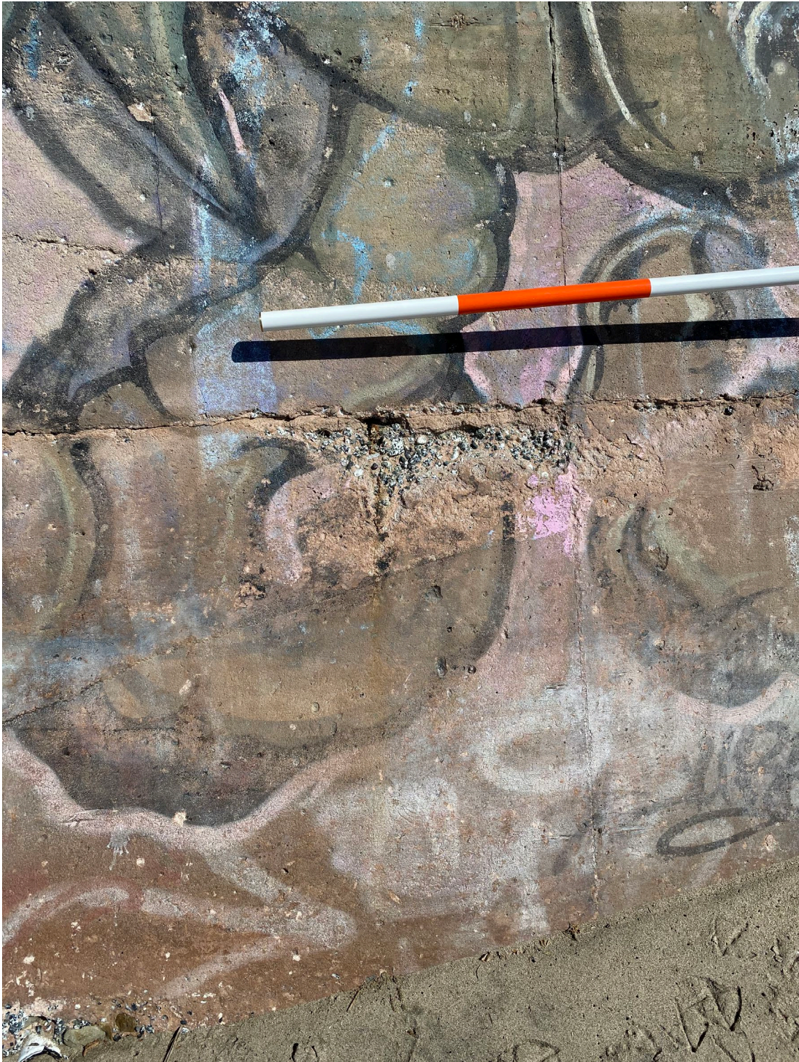
Photo 6: Close up of concrete spalling on bluff toe concrete gravity seawall - 26 May 2020
