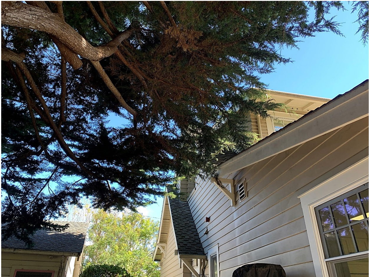
Image #7 – Note limb growth on or near neighbors roof. The limbs growing close to the home should be shortened.
