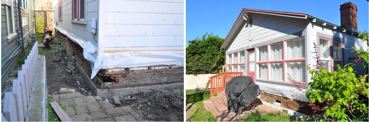
Figures 3 and 4. Left image details the south elevation, showing extensive rot to the sill plate. Right image details the west elevation, showing the deteriorated chimney and rear deck, which was replaced previously.
