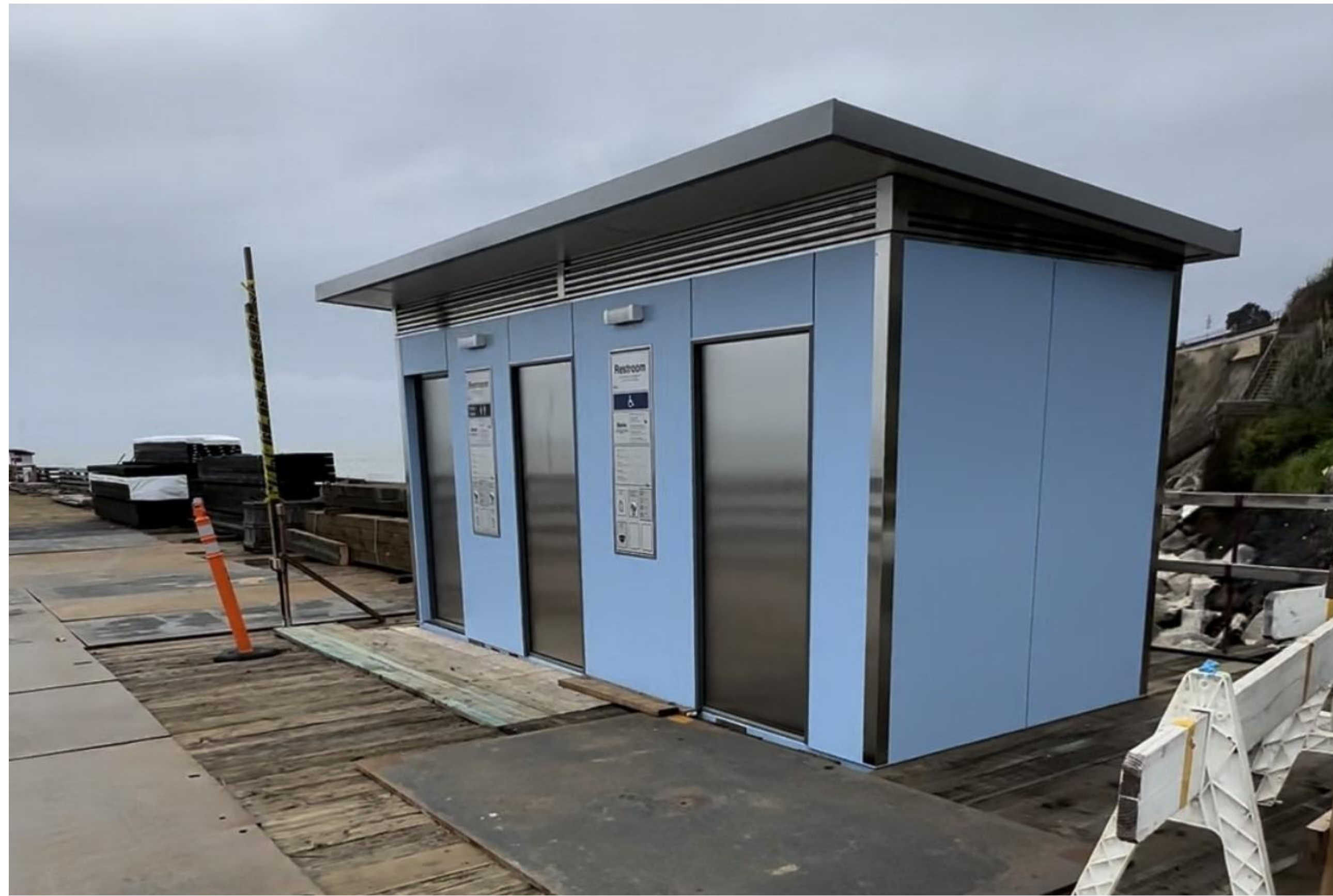
IMAGE OF THE BLUE BATHROOMS AS THEY EXIST AND ARE INSTALLED
