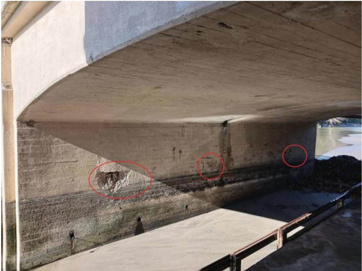
Figure 2: East Pier Wall During Very Low Tide with Spalled Areas Circled in Red
