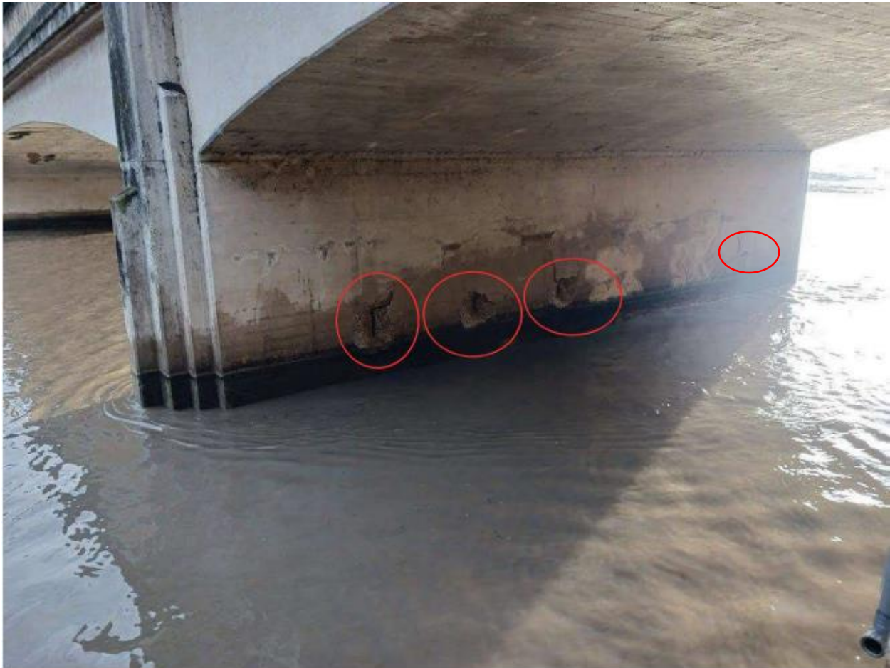
Figure 3: West Pier Wall in Post Storm Condition with Spalled Areas Circled in Red
