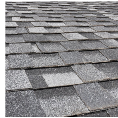
5A. COMPOSITE SHINGLE ROOF CertainTeed, Landmark Series Color: Weathered Wood
