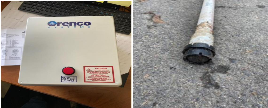
Figures 1 and 2: New replacement Orenco Panel and failing ultrasonic sensor.
