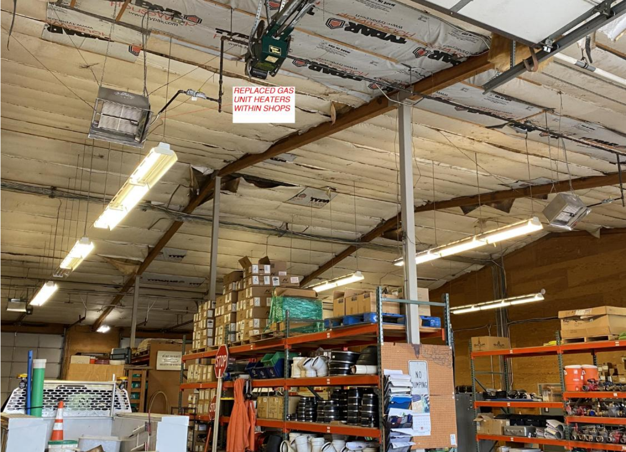
New unit heaters within maintenance garage
