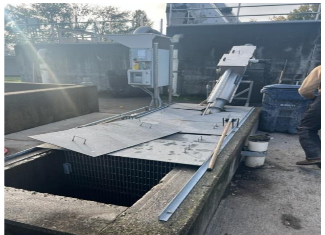
Fig. 8 Septage Receiving Station
