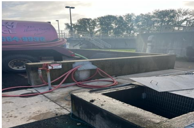
Fig 5 Septage Receiving Station
