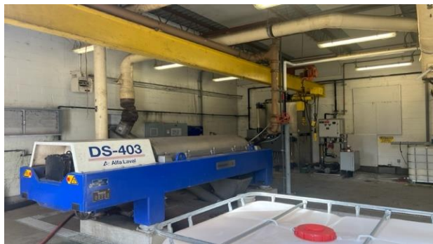
Fig.1 Centrifuge Room in Equipment bldg.
