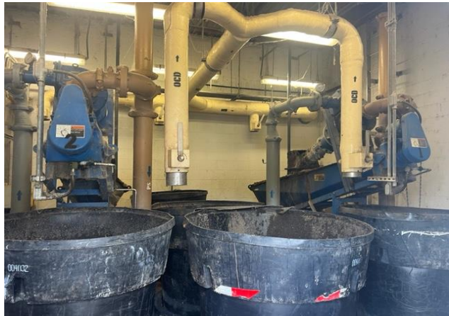
Fig.3 Grit Removal Room
