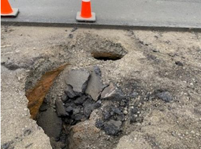
Figure 1. Sinkhole under Endicott St.
