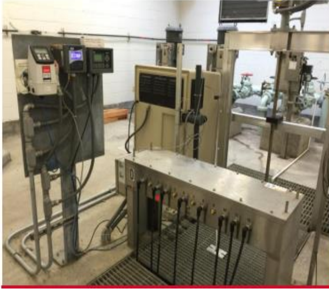
Figure 2: UV Equipment Controls
