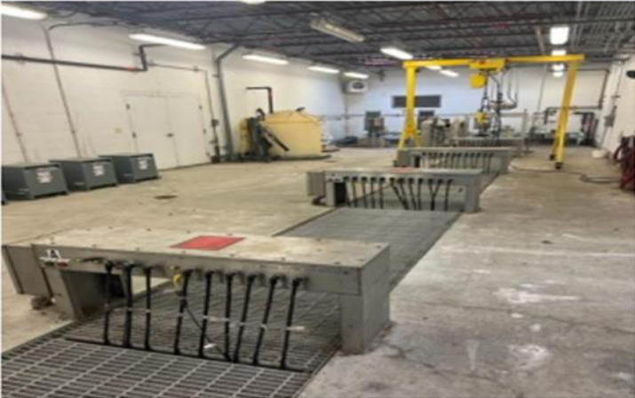
Figure 1: UV Equipment Bank
