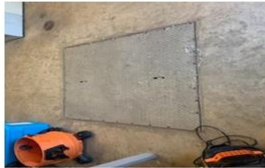
Fig 4: Substandard Hatch for Pump Access
