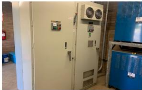
Fig 2: Variable Frequency Drive Panel
