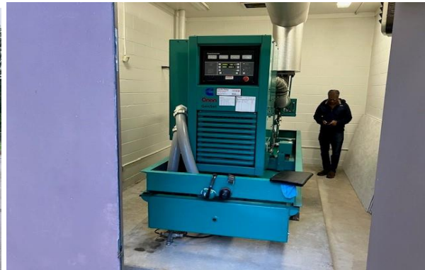
Figure 2: Angelo Booster Station Existing Generator
