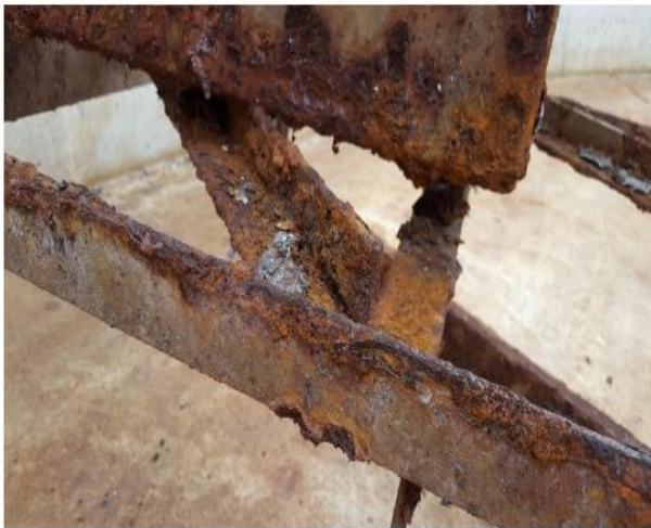
Figures 3-5: Corroded Metal in Primary Clarifier Basin
