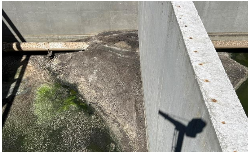
Basin #1 solids buildup
