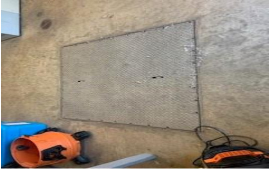
Fig 4: Substandard Hatch for Pump Access
