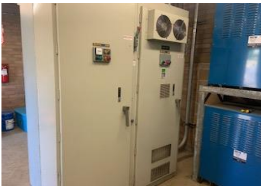
Fig 2: Variable Frequency Drive Panel
