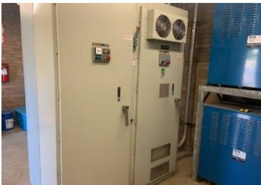
Fig 2: Variable Frequency Drive Panel
