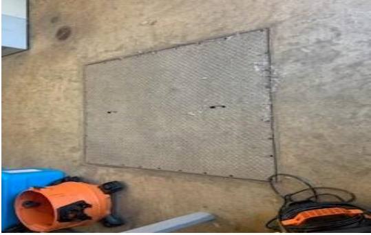
Fig 4: Substandard Hatch for Pump Access
